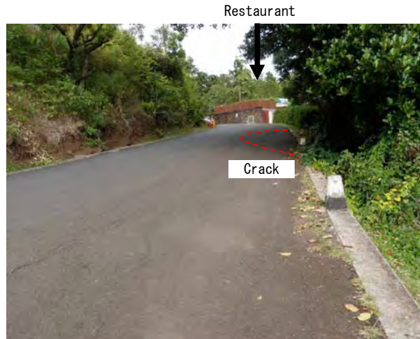
Ph-2 Crack on road side
