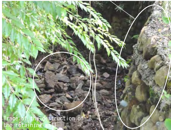
Ph-2 Trace of the destruction and the retaining wall
