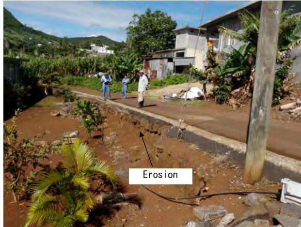
Ph-2 damage in retaining wall by erosion
