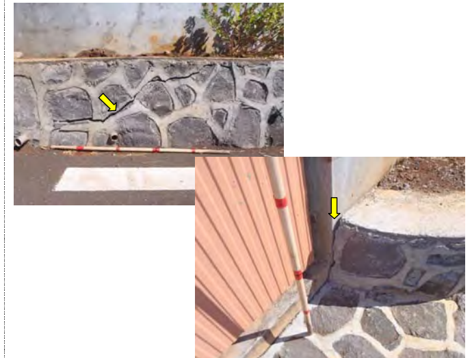
Ph-6 Cracks around the house
