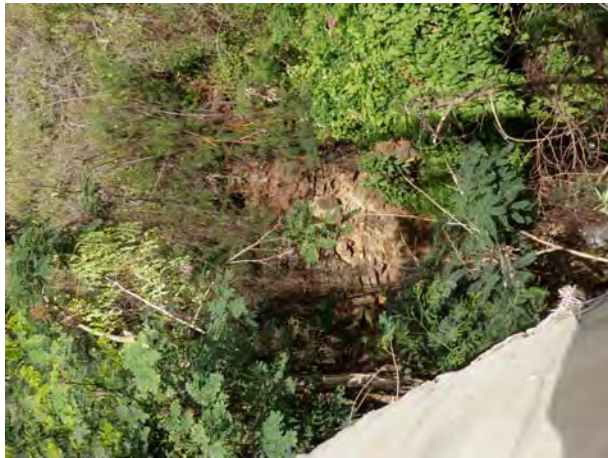
Ph-4 bank erosion
