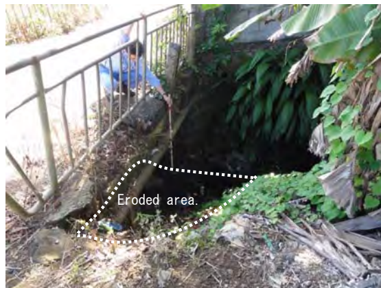
Ph-2 Eroded area
