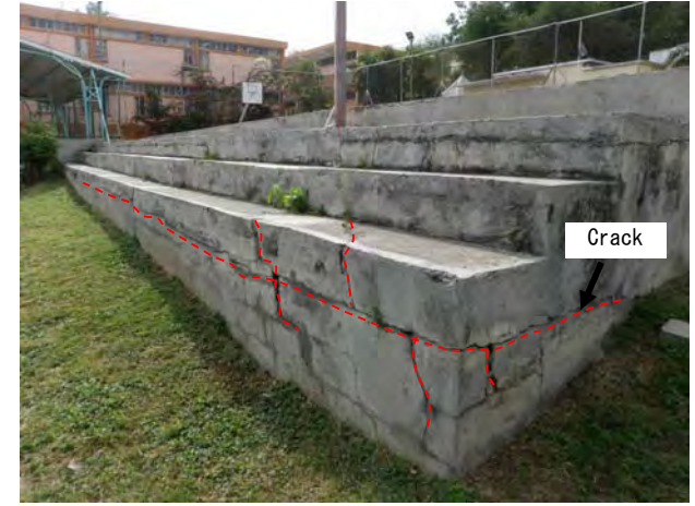
Ph-3 Horizontal crack of the Concrete step
