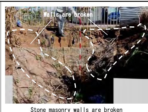
Stone masonry walls are broken
