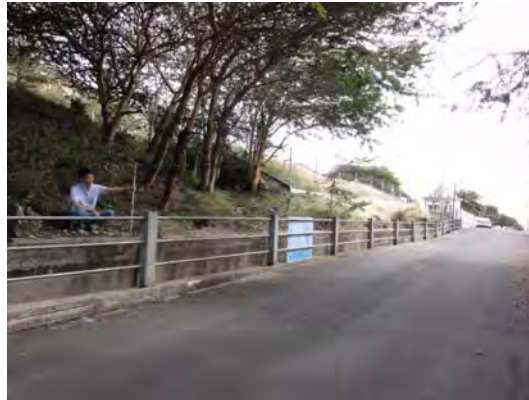
Ph-2 Slope in the retaining wall upper part
