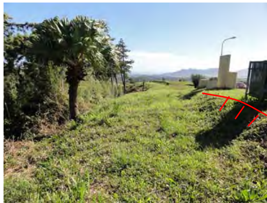
Ph-5 the around of the slope failure Topography with the Step continuously
