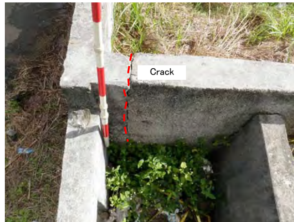
Ph-5 Crack of concrete wall
