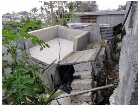
Ph-2 The broken steps
