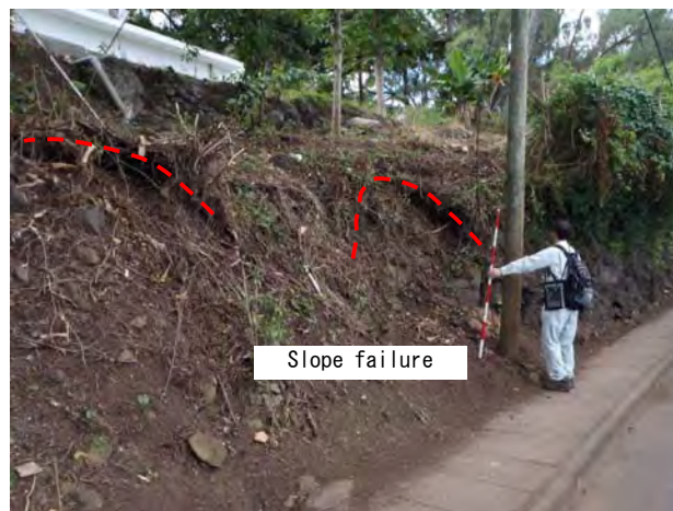
Ph-5 Surface collapse of slope
