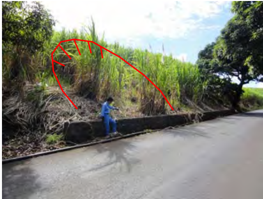
Ph-1 Full view of landslide
