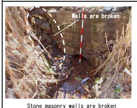
Stone masonry walls are broken
