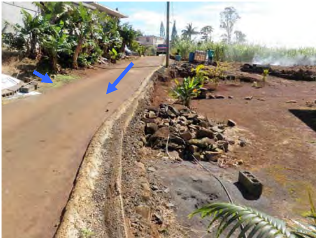
Ph-4 Retaining wall that comes off
