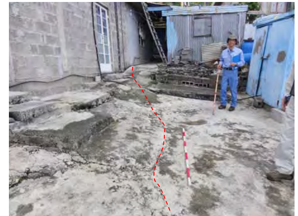
Ph-3 Observed cracks
