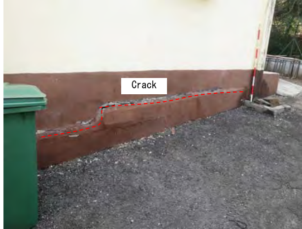
Ph-2 Cracks of wall (by differential settlement)
