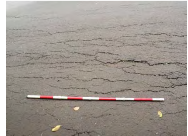
Ph-3 The crack occurred in the road sea side shoulder. (By the damage of differential settlement)
