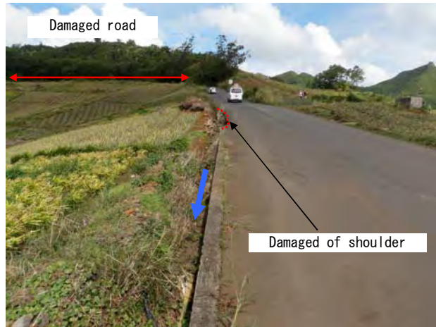
Ph-1 Full view of of damaged road
