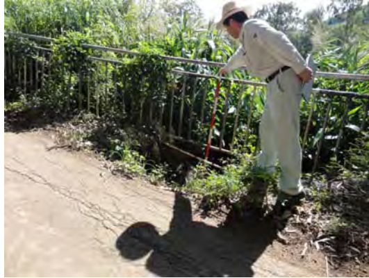
Ph-2 slope failure
