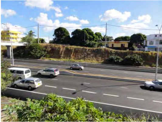
Ph-1 Full view of slope failure
