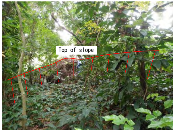
Ph-4 Slope under shoulder
