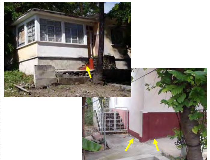
Ph-3 Damage on house
