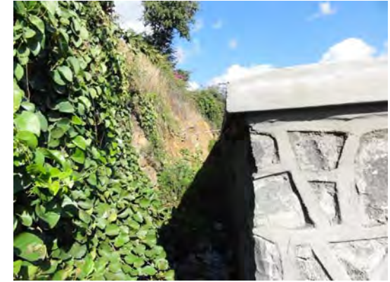
Ph-6 slope failure and retaining wall
