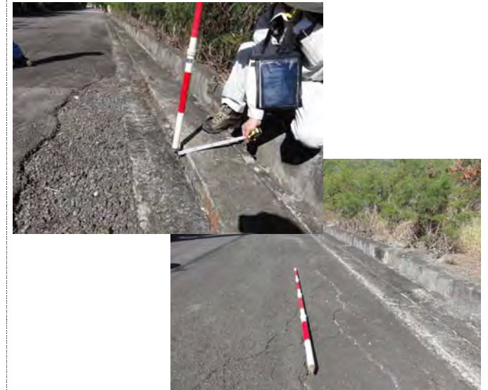
Ph-3 Cracks on the road (Upper road)
