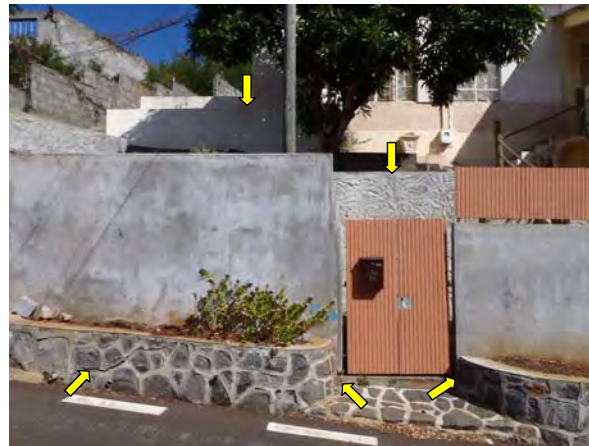
Ph-5 Damage on house
