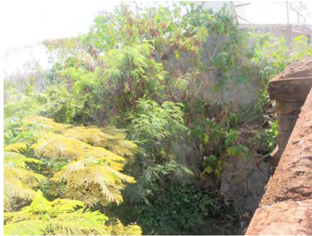
Ph-2 Bank erosion around bridge abutment
