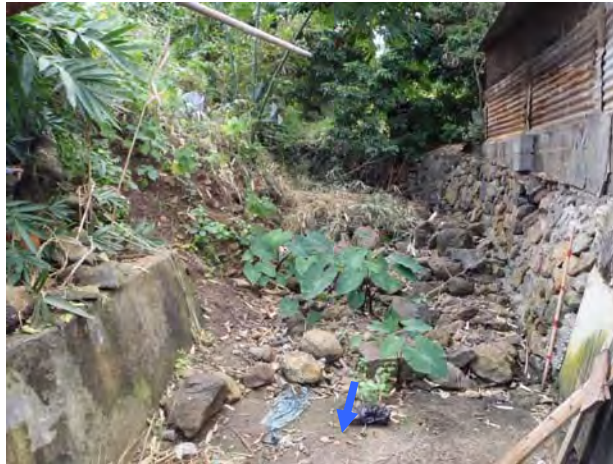
Ph-2 Unstable deposit in channel works
