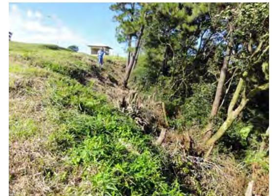
Ph-6 the around of the slope failure small slope failure
