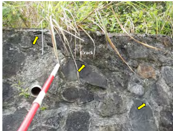
Ph-5 Cracks on retaining wall
