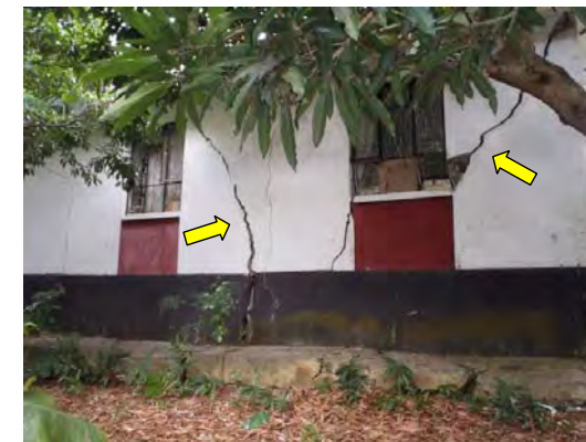
Ph-6 Damage on house (It's relocated)
