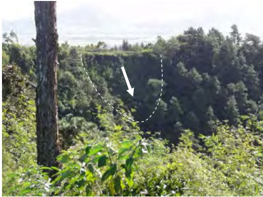
Ph-1 Full view of the slope failure
