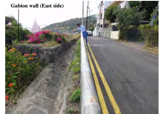
Ph-3 The upper part and the rear of the Gabion wall (East side) There is not the abnormality
