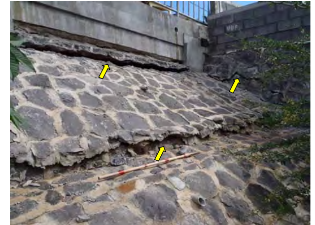
Ph-3 Cracks on Stone block
