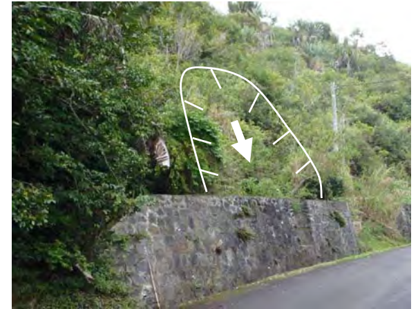
Ph-3 Trace of past slope failure
