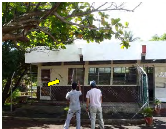
Ph-4 Damage on school (By the damage of the landslide, a part of the school cannot use)
