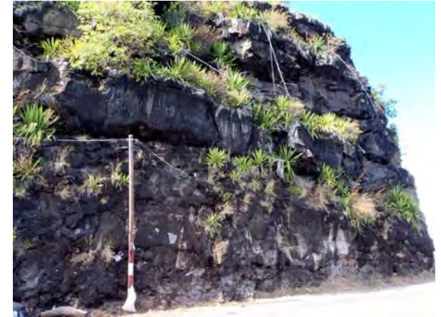
Ph-2 The rock constituting a cliff (many cracks and weathering intensely)
