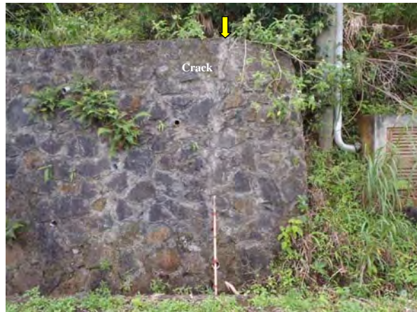
Ph-4 Cracks on retaining wall
