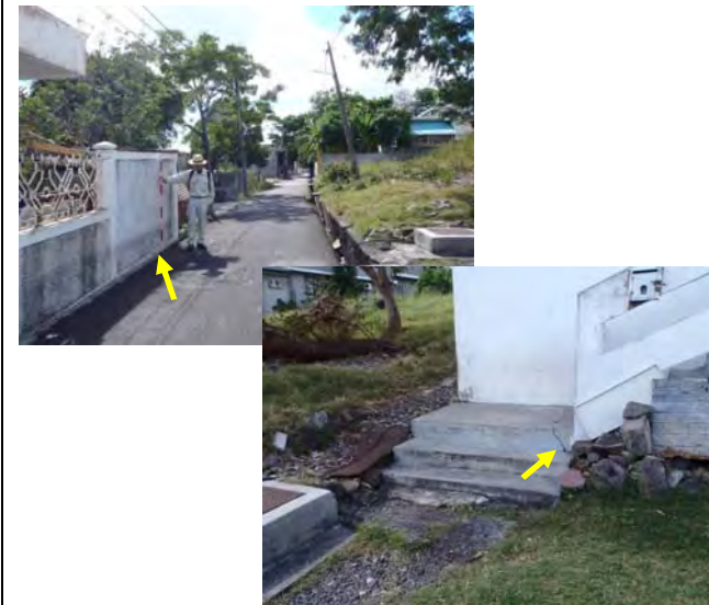
Ph-4 Damage on house
