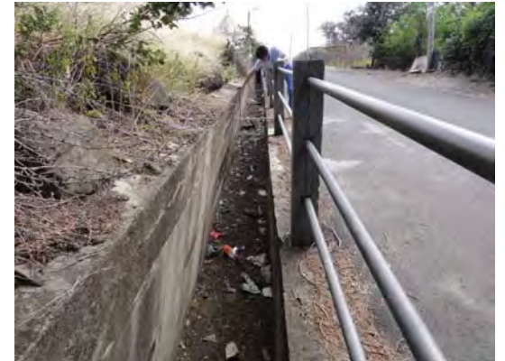
Ph-3 Inclined the retaining wall
