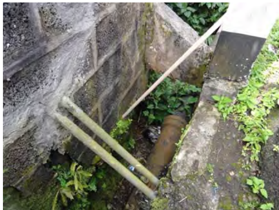
Ph-4 Eroded area The eroded depth is 50cm
