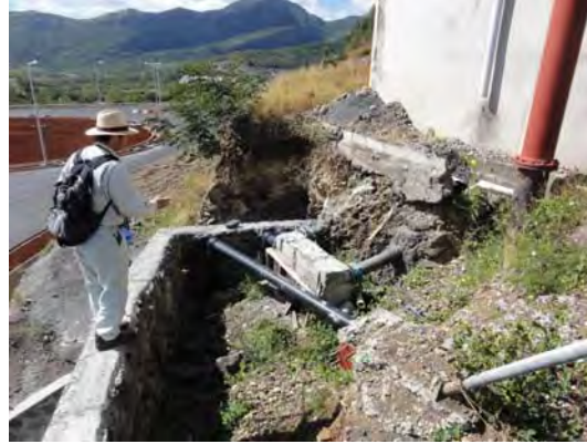
Ph-2 erosion of the groundwork
