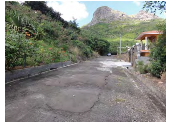
Ph-6 Cracks on the road (Lower road)
