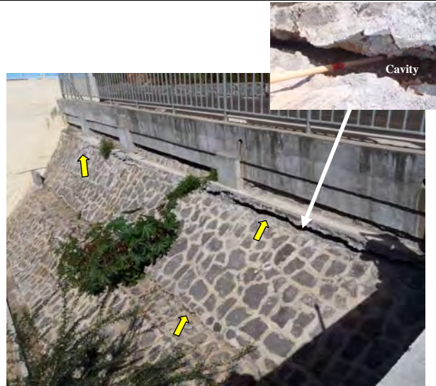
Ph-2 Cracks on Stone block
