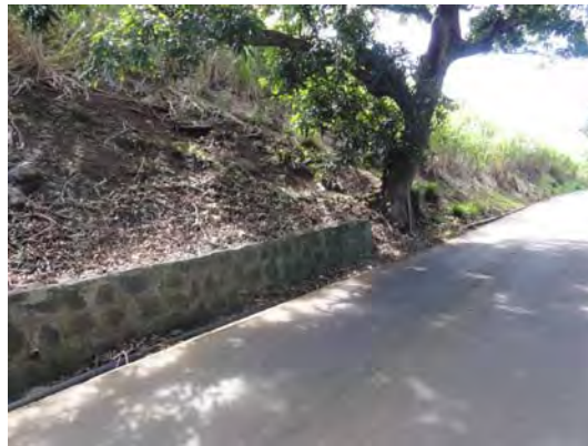
Ph-5 slope failure
