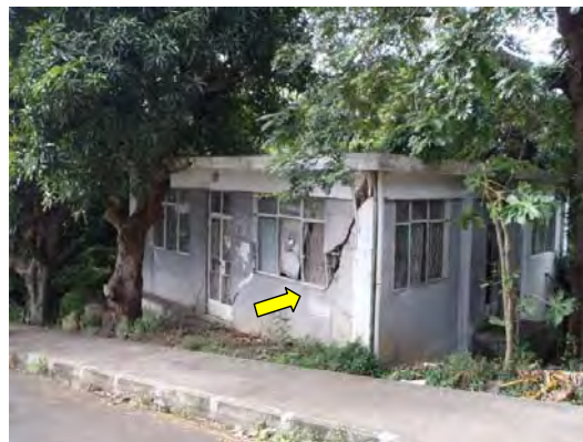
Ph-5 Damage on house (It's relocated)
