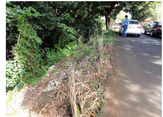
Ph-6 rocks and gravel by slope failure
