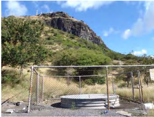
Ph-1 Drainage Well (W-2)
