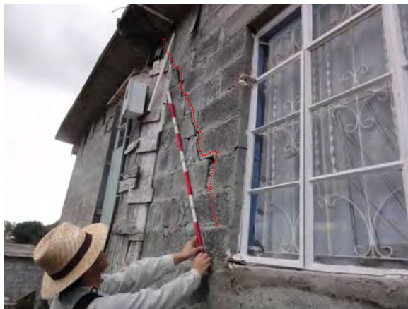
Ph-4 Damage on house (Caused by landslide)
