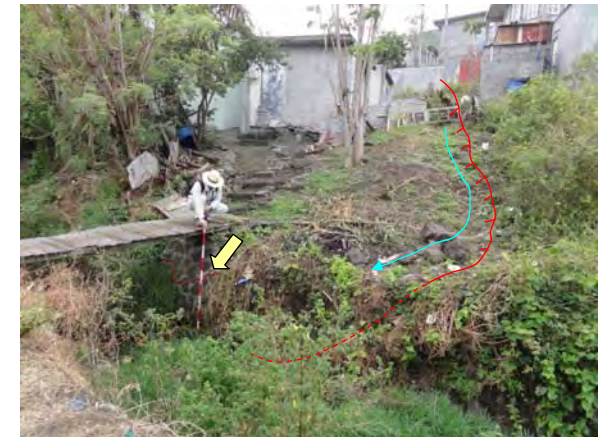
Ph-6 Cracks at bank protection
