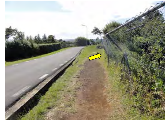
Ph-3 the fence in the back of slope failure It is damaged by slope failure
