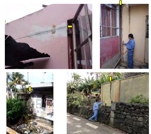
Ph-6 Heavy damage on house
