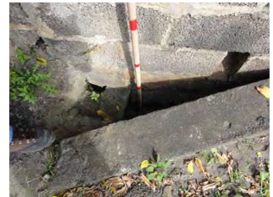
Ph-5 Damage of the drainage of the roadside
