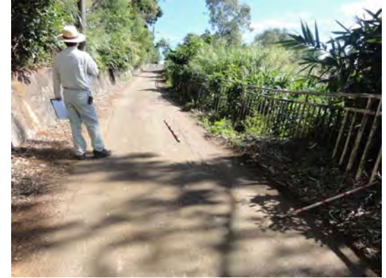
Ph-3 Transverse Cracks
