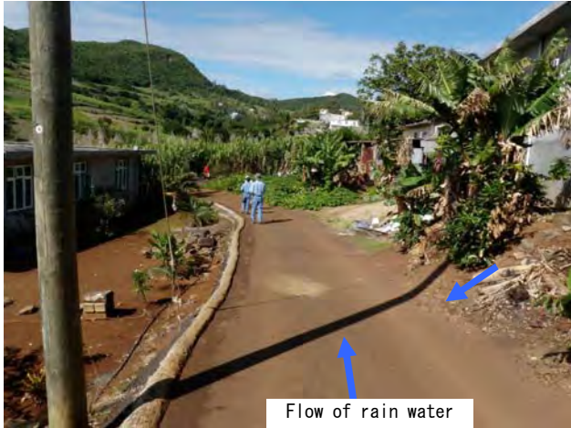
Ph-1 Full view of damage of retaining wall
