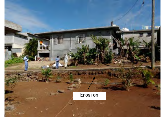
Ph-3 damage in retaining wall by erosion
