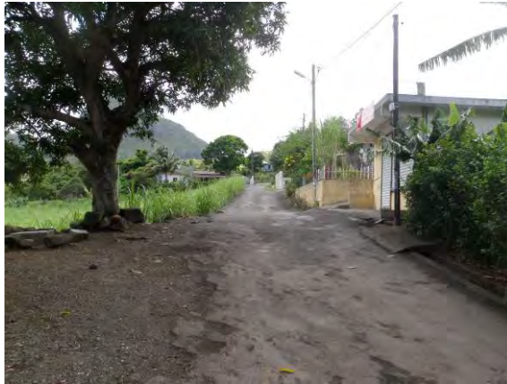
Photo 3.7.47 Cracks in the Road (Left: Sugarcane Field)
