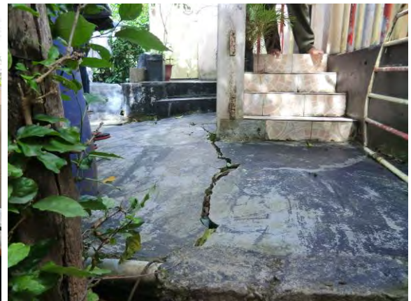
Photo 3.7.80 Open Cracks in the Foundation
