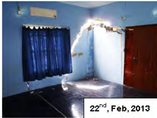
Photo 3.7.95 Open crack in the room of House (1) (source:JET)
