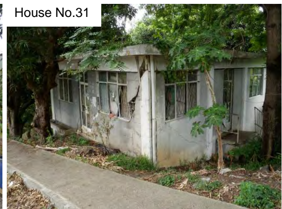
House No.31 Photo 3.7.32 Penetrating Cracks in the Wall
