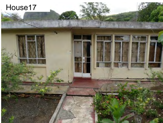
Photo 3.7.19 Heavily Damaged House
