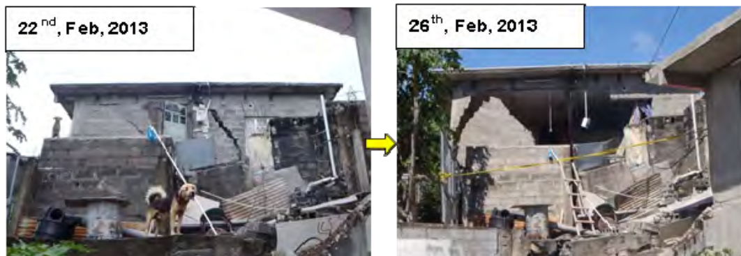
Photo 3.7.97 The Outside Wall of House (1) was Completely Broken (source:JET)
