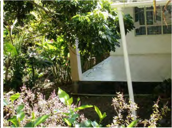
Photo 3.7.24 Cracks in the Veranda
