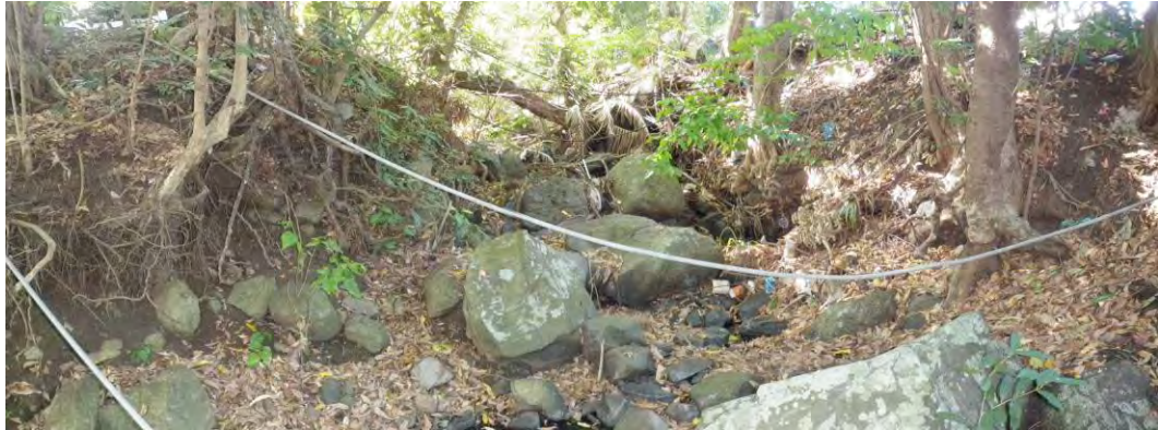
Photo 3.7.44 Advancement of Bank Erosion (Upstream) (source:JET)
