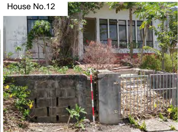
Photo 3.7.46 Open Cracks in the House and Retaining Wall
