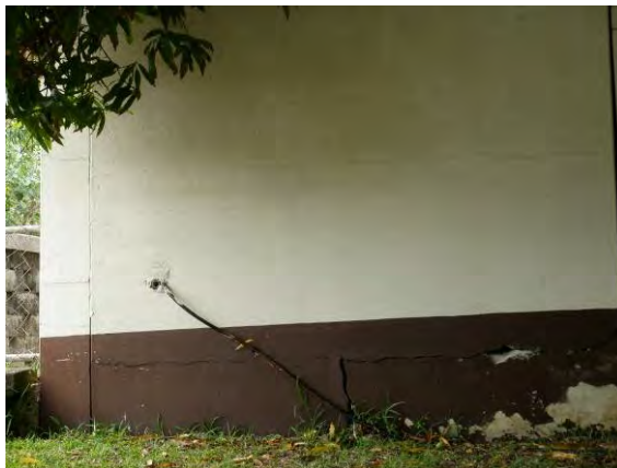
Photo 3.7.16 Cracks in the Base of the Wall
