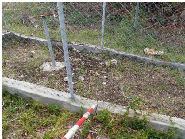
Photo 3.7.39 Deformation of the Protection Fence foundation (source:JET)
