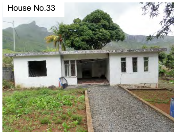
House No.33 Photo 3.7.31 Inclination of the House (Left: Settling)
