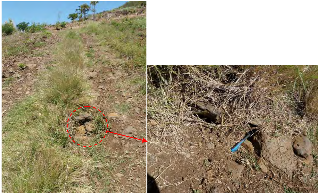
Photo 3.7.70 Cracks along the Farm Road (source:JET)
