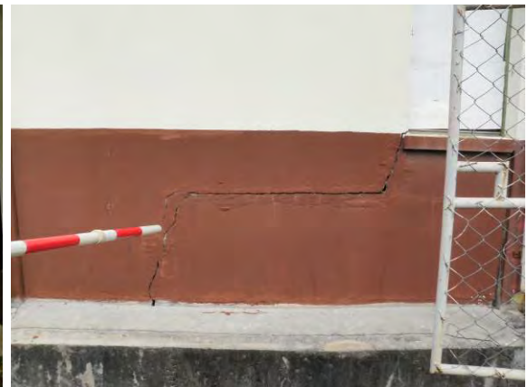
Photo 3.7.17 Cracks in the corner of the School Building
