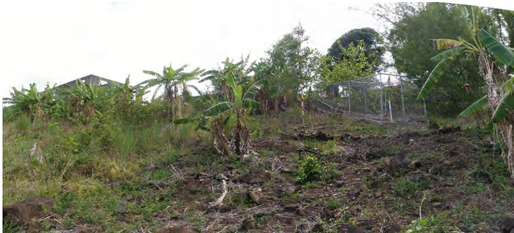
Photo 3.7.38 Extensometer E(2) (Shot from below) (source:JET)
