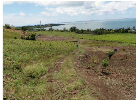
Photo 3.7.69 Cracks in the Farm Road (from above) (source:JET)
