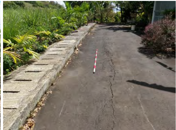
Photo 3.7.75 Cracks in the Road
