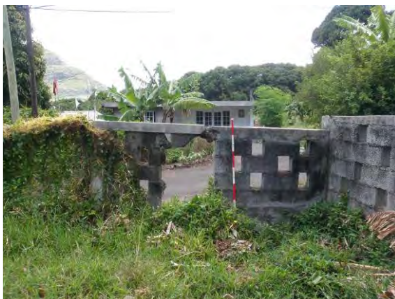
Photo 3.7.11 Damage to the Retaining Wall (Roadside)
