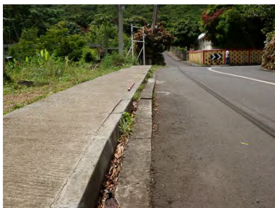
Photo 3.7.21 Gaps and Unevenness in the Curb
