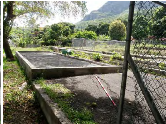
Photo 3.7.8 Intermittent Cracks (East-West)
