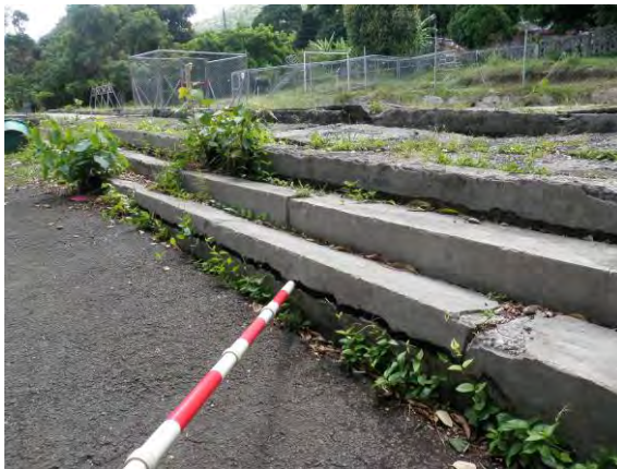
Photo 3.7.7 Major Damage to the Steps
