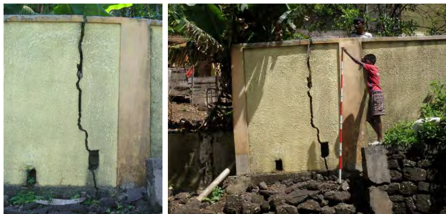
Photo 3.7.86 Cracks in the Concrete Wall (Left: 2011, Right: Present) (source:JET)
