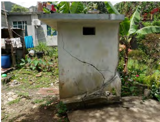
Photo 3.7.27 Cracks in the Concrete Structure
