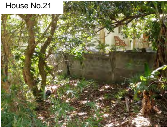
Photo 3.7.23 Cracks in the Retaining Wall beside House
