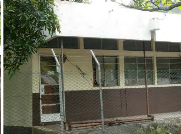
Photo 3.7.15 Cracks in the School Wall
