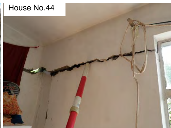
Photo 3.7.37 Horizontal Open Cracks
