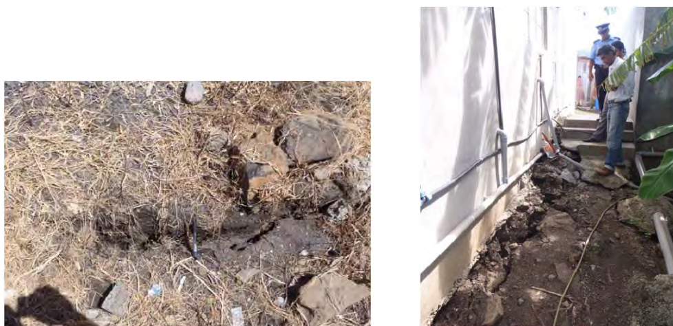
Photo 3.7.98 New Open Cracks in the Upper Part of House (1) (source: JET)
