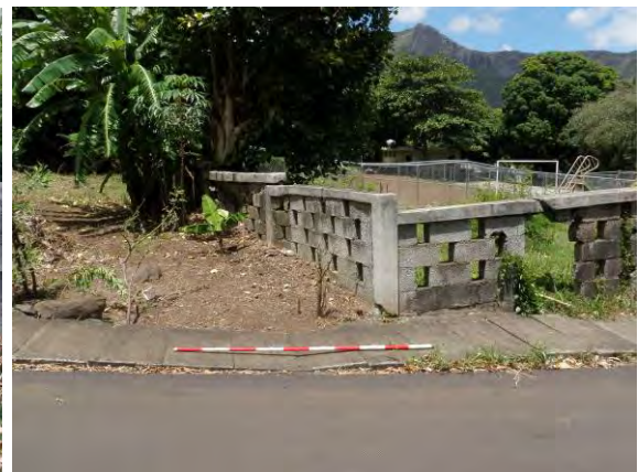
Photo 3.7.12 Settling of the Roadside Ditch
