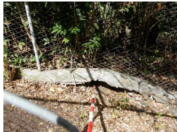
Photo 3.7.35 Deformation of the Protection Fence Foundation Concrete (source:JET)
