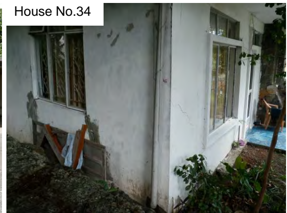
House No.34 Photo 3.7.30 Cracks in the Wall (Window Frame)
