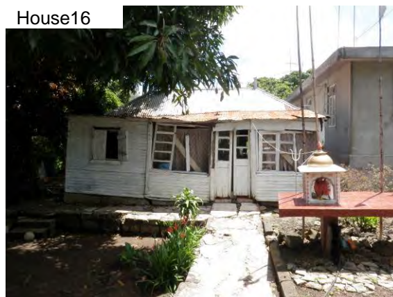
Photo 3.7.20 Heavily Damaged House
