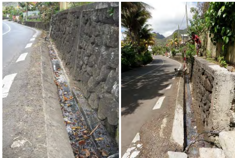
Photo 3.7.85 Swelling on the Road (Left: 2011, Right: Present) (source:JET)
