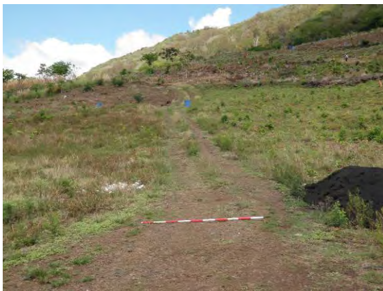
Photo 3.7.68 Cracks in the Farm Road (from below)
