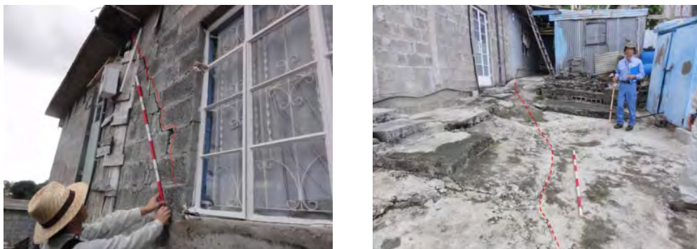
Photo 3.7.89 Damage to House (1) (source: JET)
