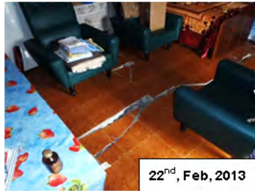
Photo 3.7.96 The cracks and steps in the room of House (1) (source:JET)
