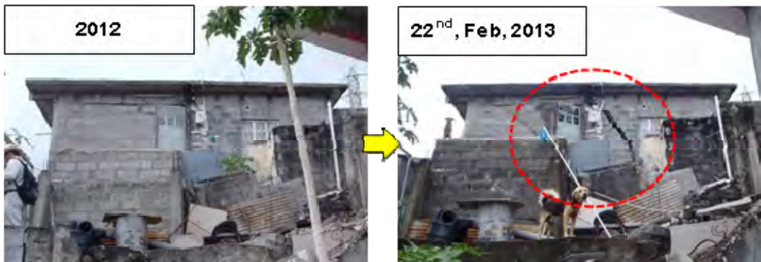
Photo 3.7.93 Damage on the Outer Wall of House(1), Large Open Crack Grew (source: JET)
