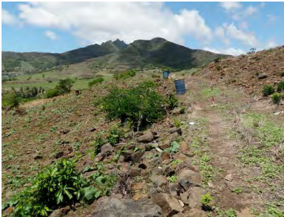
Photo 3.7.66 Deformations around Borehole BH-1 (Current Condition)
