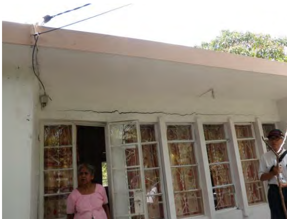
Photo 3.7.79 Horizontal Open Cracks in the Wall
