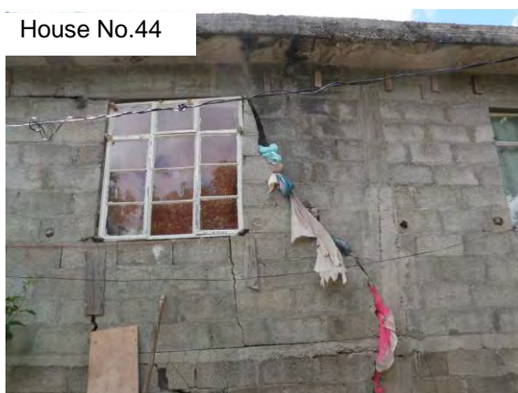
Photo 3.7.36 Cracks in the House Wall
