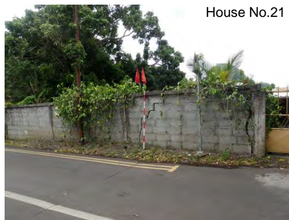
Photo 3.7.22 Cracks in the Retaining Wall of the House in front of the School (source:JET)
