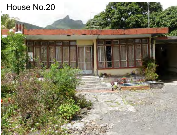
House No.20 Photo 3.7.29 Settling in the Middle of House
