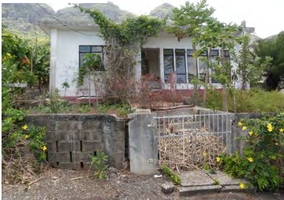
Photo 3.7.45 Heavily Damaged House
