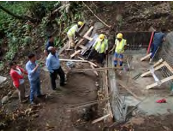
2 nd Site Meeting for the Construction of Landslide Countermeasure Works (Chitrakoot), 1 st Sep. 2014
