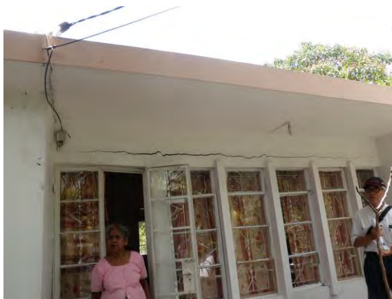
Photo 3.7.3 Horizontal Open Cracks in the Wall
