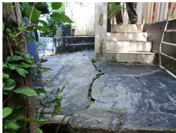
Photo 3.7.4 Open Cracks in the Foundation
