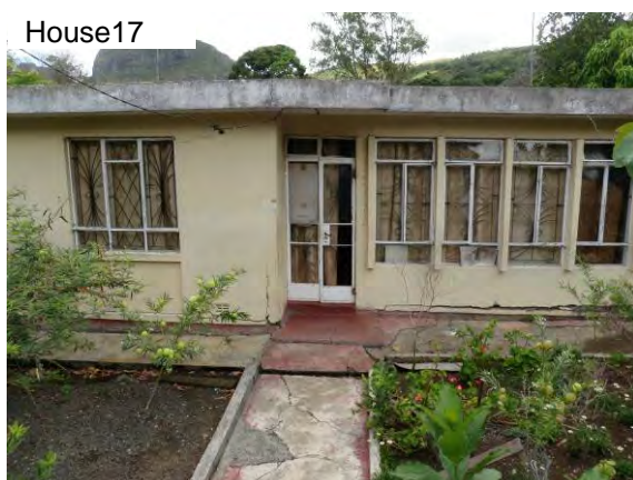
Photo 3.7.1 Heavily Damaged House
