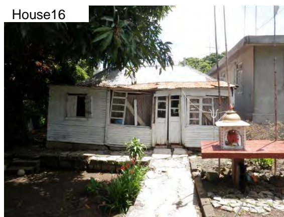
Photo 3.7.2 Heavily Damaged House
