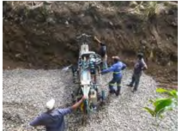
Technical Guidance on Horizontal Drilling for Landslide Countermeasure Works (Chitrakoot), 30 th Oct. 2014
