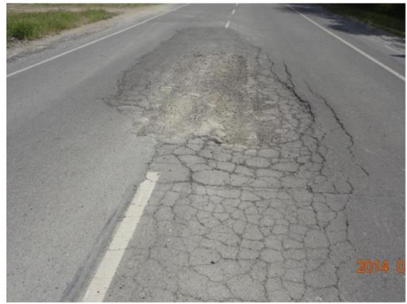
Alligator Crack on AC Pavement/ Exposure of AS Stabilized Base Course
