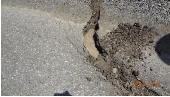
Crack Opening Section
