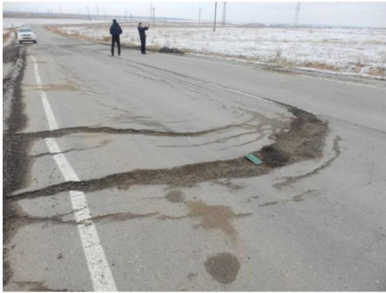
Sliding of AC Pavement
