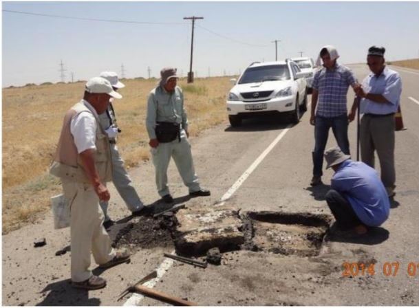
Survey of Adhesion between AC Pavement and Cement-Stabilized Base Course on Steep Section
