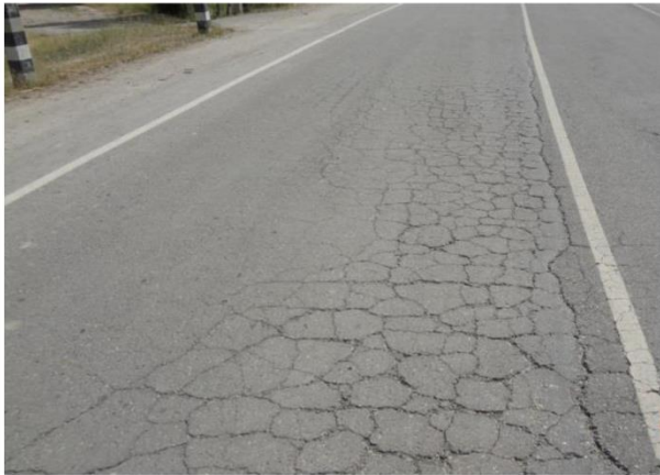
Alligator Crack on AC Pavement
