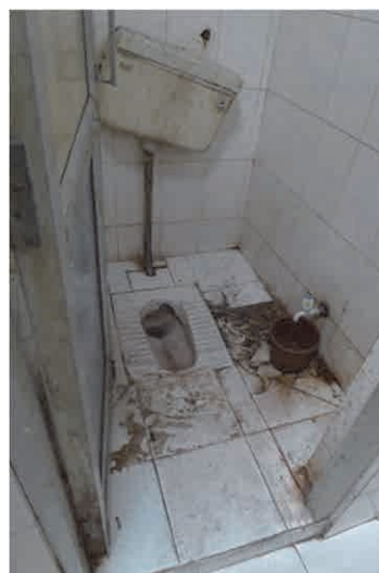
Conditions of facilities are poor
