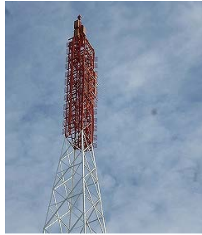
MBCo: Antenna Tower
