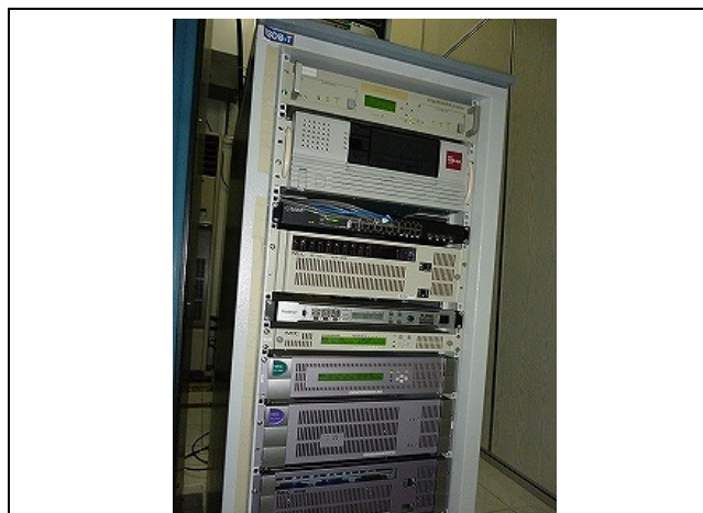
MBCo: ISDB-T Transmitter
