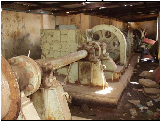
Photo C.2.17 No.6 Hauling Winch
