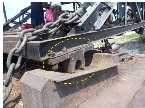
Photo 5 - Roller wheel is missing
