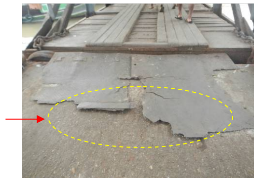
Photo 6 - Bridge facility damage
