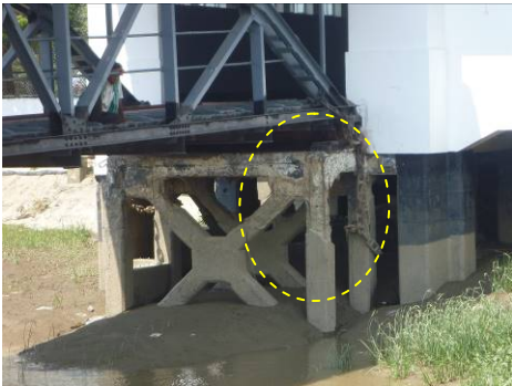
Photo 2 - Abutment column damage
