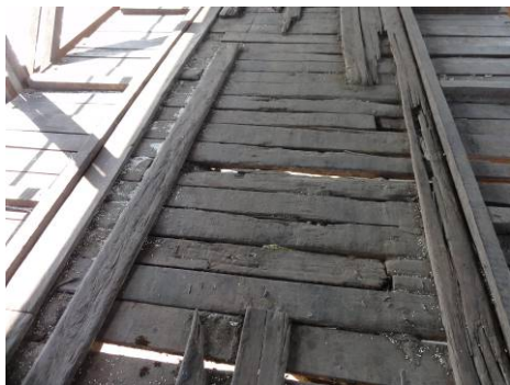
Photo 3 - Timber decking loss & damage
