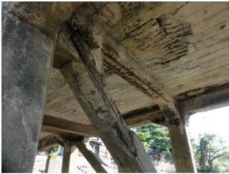
Photo 2 - Beam , slab rebar exposed and rusted
