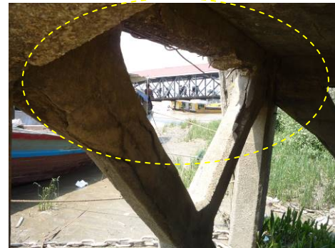
Photo 6 - Seriously damage the beams and bracing
