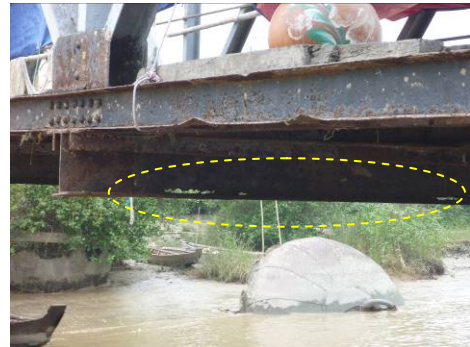
Photo 5 - Member is rusted and damage
