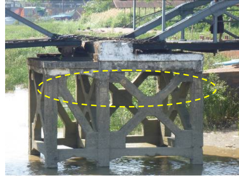
Photo 4 - Abutment column and bracing damage
