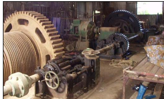
Photo C.2.4 No.2.3 Hauling Winch
