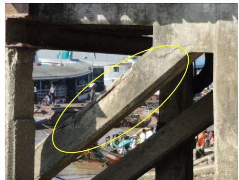
Photo 7 - Pier bracing defected
