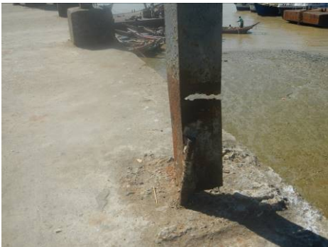
Photo 2 - Hand rail Post damage
