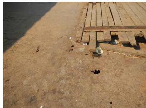
Photo 6 - Hole at Pontoon surface
