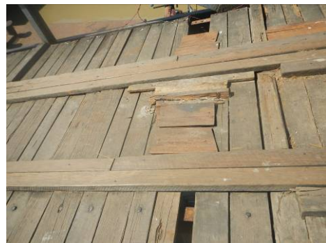
Photo 6 - Timber Decking damage
