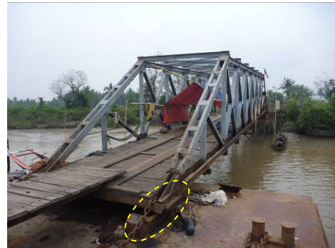
Photo 4 - Roller wheel is missing
