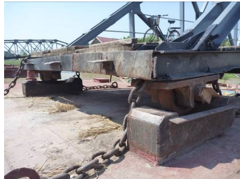
Photo 5 - Roller wheel missing
