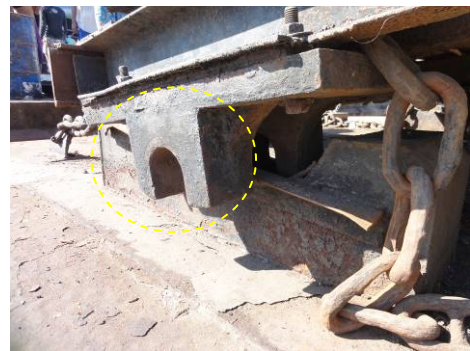
Photo 9 - Roller wheel is missing
