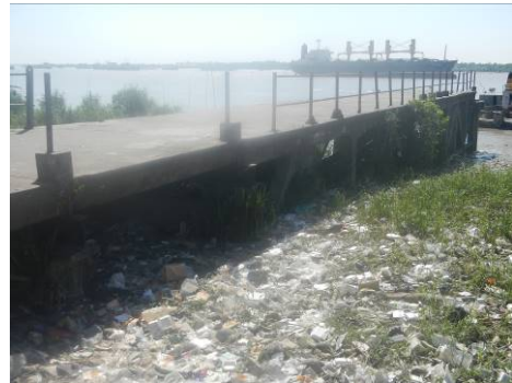
Photo 3 - Hand rail missing
