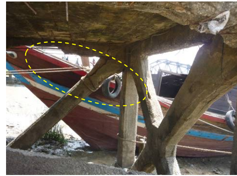
Photo 5 - Bracing & Column damage
