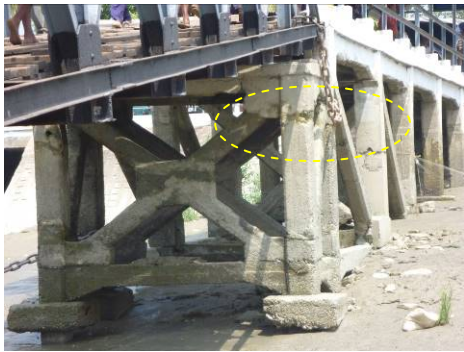
Photo 2 - Abutment column damage
