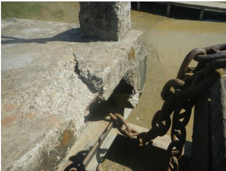
Photo 2 - Slab corner damage
