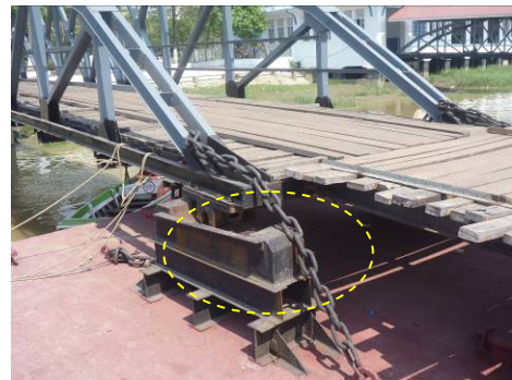
Photo 5 - Roller wheel missing
