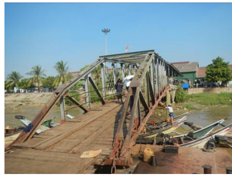
Photo 4 - Decking timbers lost
