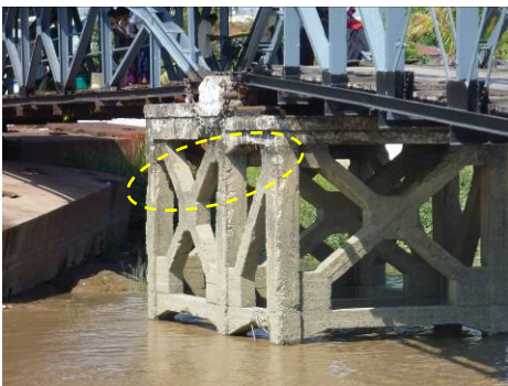
Photo 3- Abutment column damage
