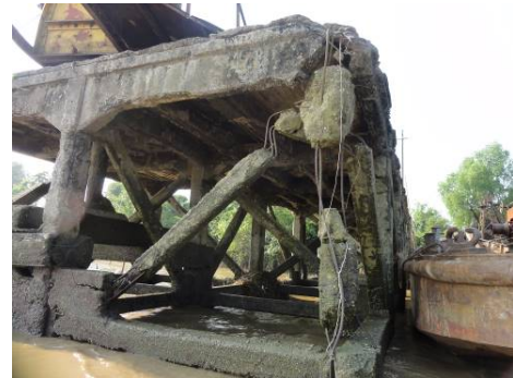
Photo 5 - Column and bracing are totally damage
