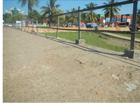
Photo 4 - Hand rail post damage
