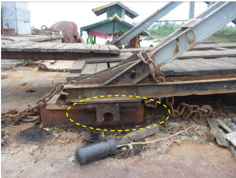
Photo 2 - Roller wheel is missing,
