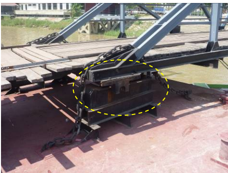
Photo 3 - Roller wheel is missing
