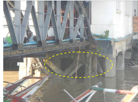
Photo 4 - Abutment Column Damage
