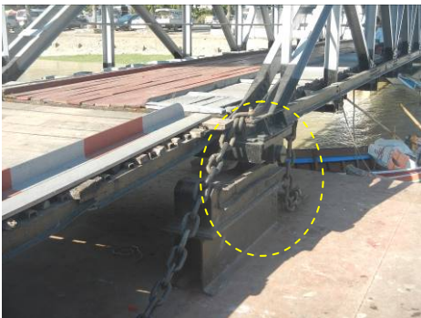
Photo 2 - Roller wheel is missing
