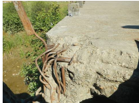
Photo 5 - Damage corner of Abutment
