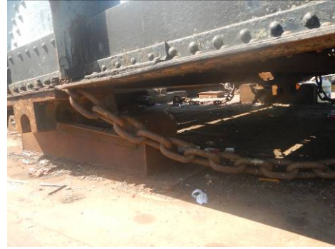
Photo 8 - Roller Wheel missing
