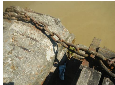
Photo 5 - Abutment concrete damage
