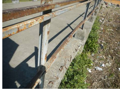
Photo 4 - Corner rebar expose
