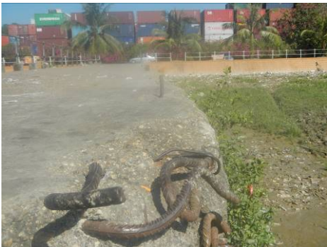
Photo 2 - Edge of Concrete Slab damage
