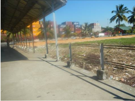
Photo 9 - Hand rail missing
