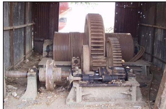
Photo C.2.8 No.7-12 Hauling Winch
