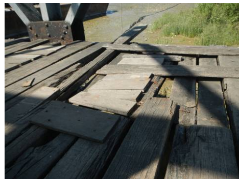
Photo 6 - Timber Decking Damage
