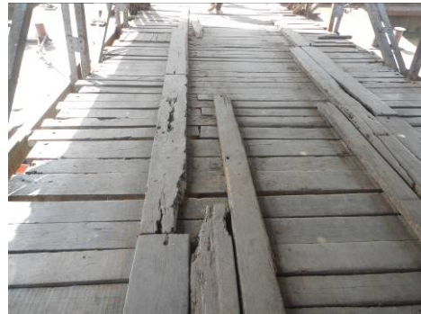
Photo 5 - Timber decking loss
