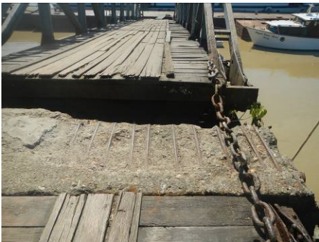
Photo 2 - Abutment Slab concrete damage
