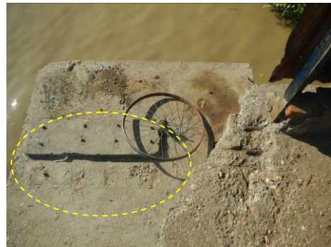
Photo 4 - Abutment slab corner damage
