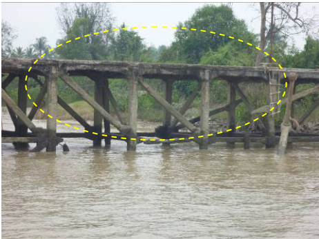
Photo 2 - Beams and bracings are totally damage
