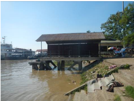
Photo 2 - Abutment slab corner damage
