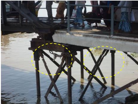
Photo 2 - Support is rusted & broken
