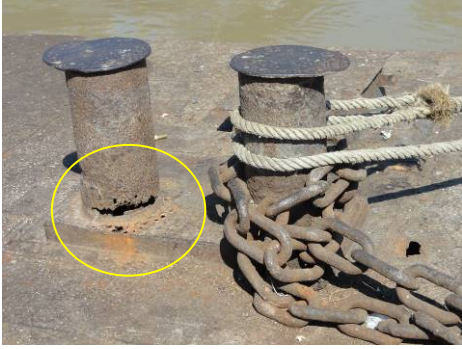
Photo 7 - Bollard base damage
