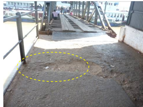
Photo 4 - Passenger way is damage
