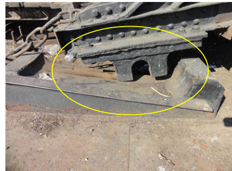
Photo 5 - Roller wheel is missing
