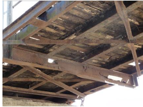
Photo 4 - Porter way girder rust and damage
