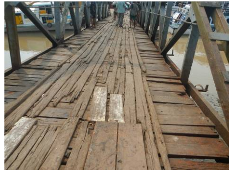
Photo 5 - Timber loose & damage
