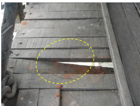
Photo 3 - Decking timber loose
