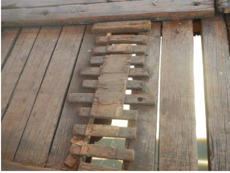
Photo 7 - Timber decking damage
