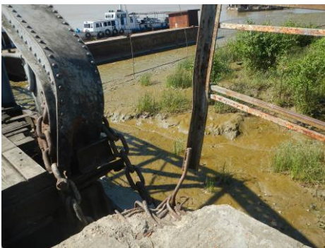
Photo 3 - Corner damage, Rebar expose
