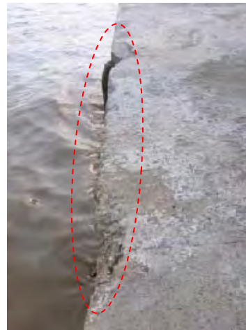
Photo 5 - Flaking of concrete
