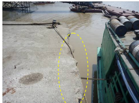
Photo 5 - Concrete slab damage
