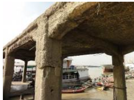
Photo 6 - Beam damage, Rebar is exposed
