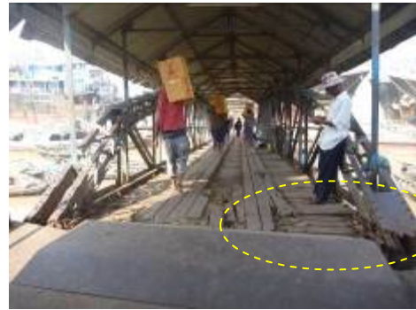
Photo 4 - Decking timber lost
