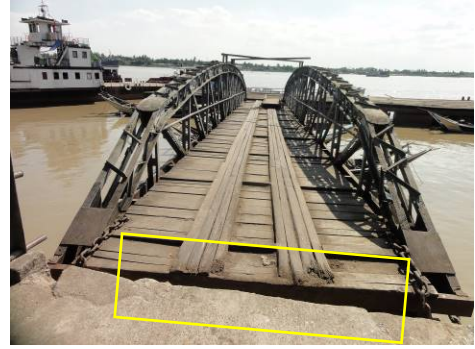
Photo 7 - Connection cover steel plate missing
