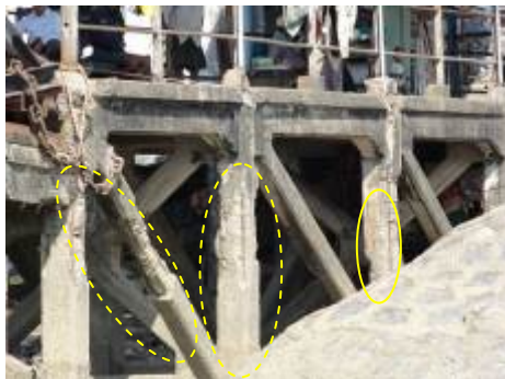
Photo 2 - Bracing & Colum damage
