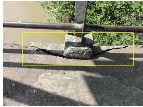
Photo 4 - Hand rail post damage
