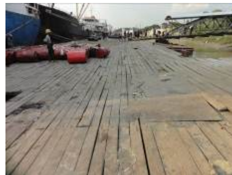
Photo 5 - Deck timber lost
