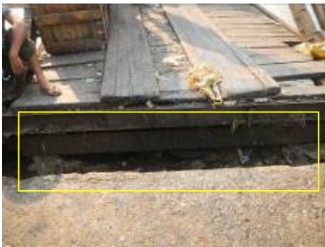
Photo 2 - Connection cover plate missing
