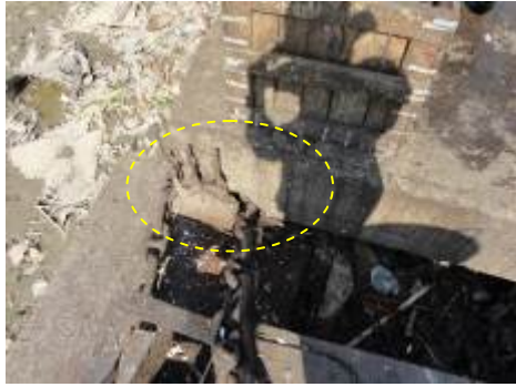
Photo 3 - Corner of Pier Concrete slab damage
