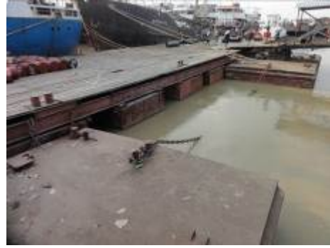
Photo 6 - Decking support beam rusted, need to replace
