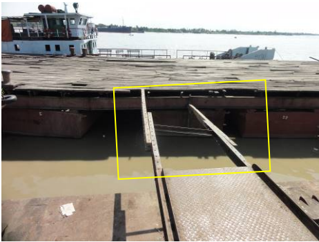
Photo 2 - No connection with Pontoon
