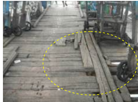
Photo 5 - Timber decking damage
