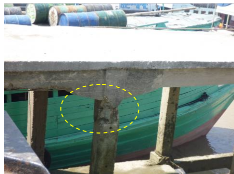
Photo 6 - Pier column damage
