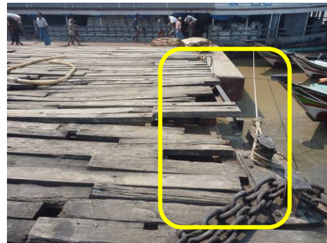
Photo 6 - Timber decking loss & damage
