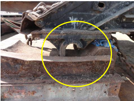
Photo 2 - Roller wheel is missing
