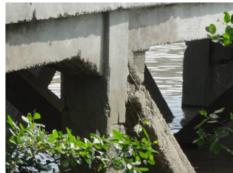
Photo 5 - Pier concrete damage
