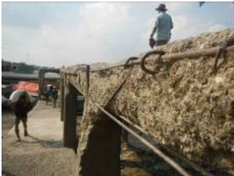
Photo 2 - Concrete column and slab damage
