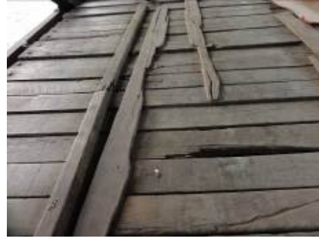
Photo 6 - Decking Timber loss & damage
