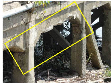
Photo 5 - Pier column & beam damage
