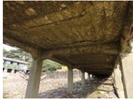
Photo 5 - Beam & slab damage
