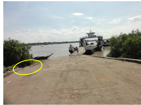
Photo 3 - Curb Stone Damage
