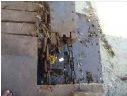
Photo 2 - Bridge roller connection rusted
