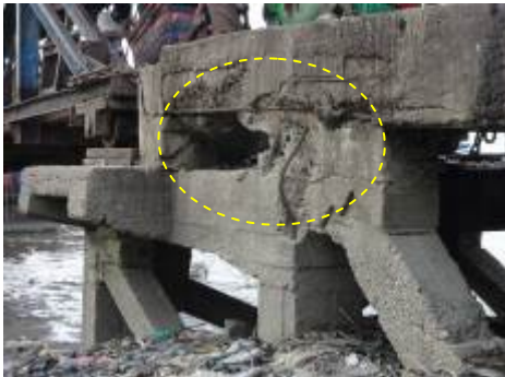
Photo 2 - Pier concrete damaged
