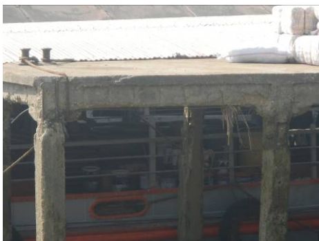
Photo 3 - Beam, column & slab damage
