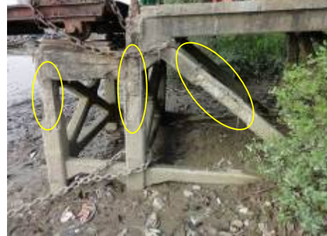
Photo 8 - Bracing & Colum damage
