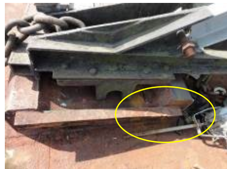
Photo 5 - Roller Wheel Missing
