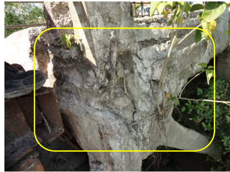
Photo 5 - Porter Way Damage, rebar export and rust
