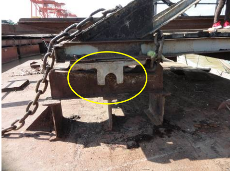
Photo 4 - Roller wheel missing
