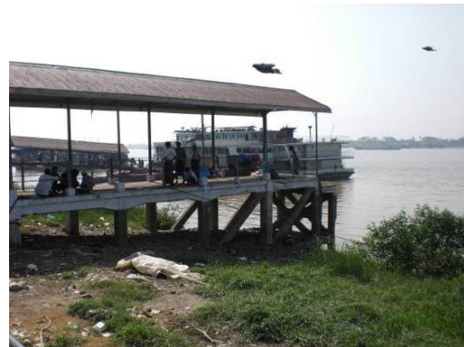
Photo 6.2 Damaged Phoneygilan Jetty
