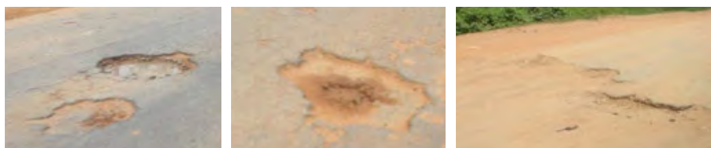
Figure 4.1 Potholes and Pavement Failure
