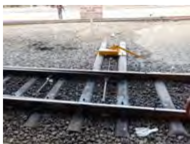
Manually operated Switching device
