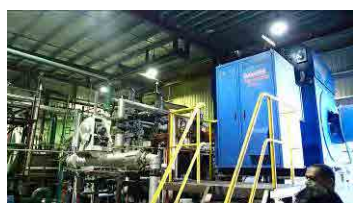
Turbine and generator
