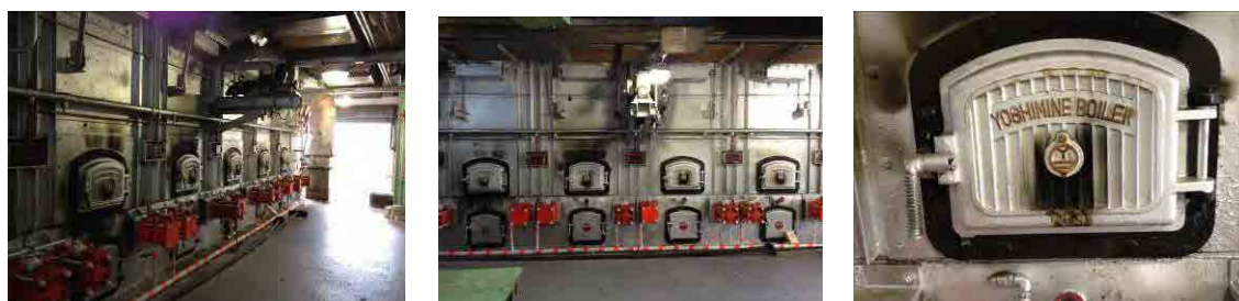
Boiler (Yoshimine; JAPAN)
