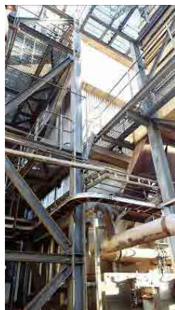
Boiler (Yoshimine; Japan)
