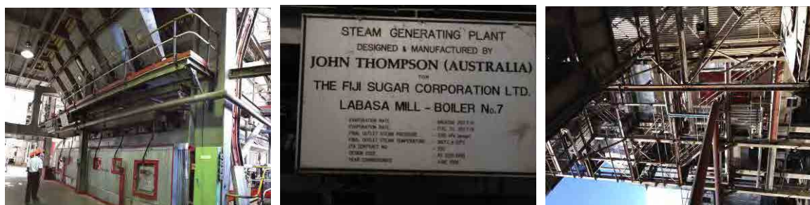
Boiler (Yoshimine; JAPAN)
