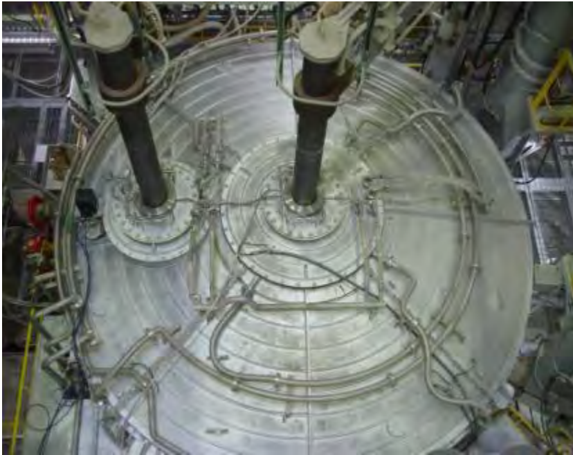
ash melting furnace
