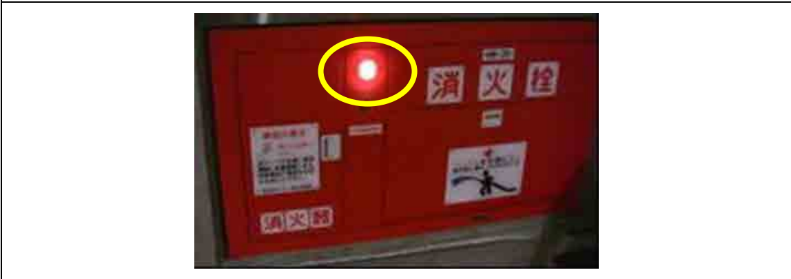
Push Button Alarm with Extinguisher & Fire Hydrant
