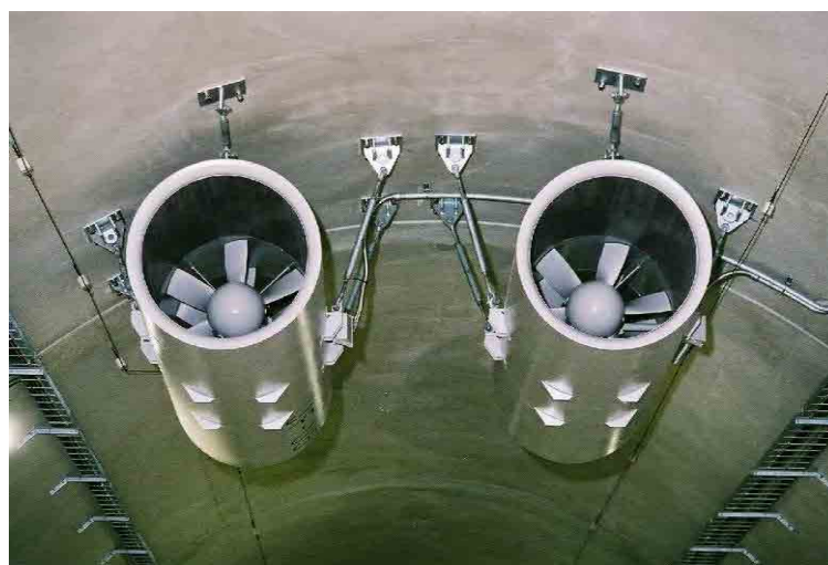
PHOTO 9.9-1 JET FANS INSIDE TUNNEL
