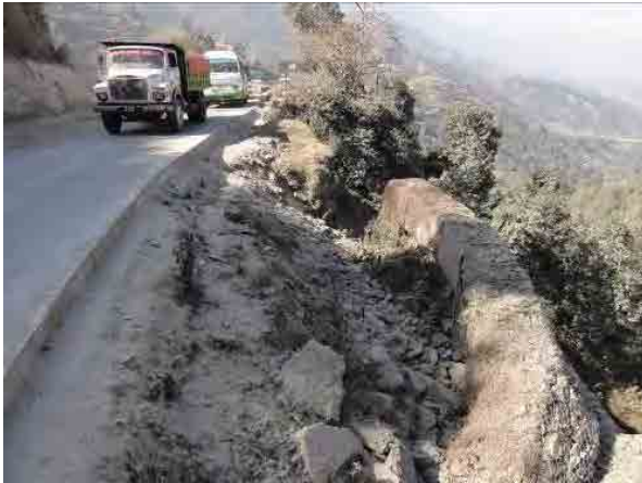
FIGURE 6.2-9 COLLAPSE OF ROAD SHOULDER
