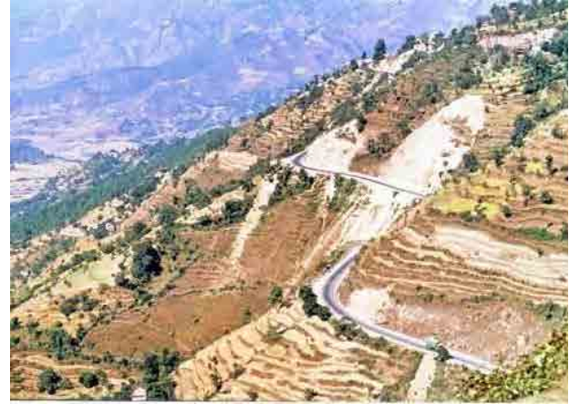
FIGURE 6.2-10 CUTSLOPE COLLAPSE AFTER HARD RAINFALL
