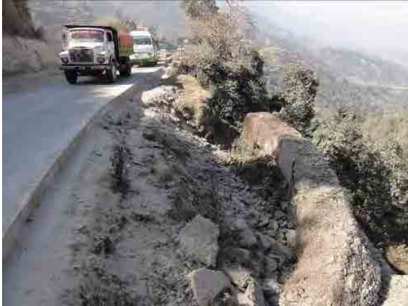
FIGURE 6.2-9 COLLAPSE OF ROAD SHOULDER
