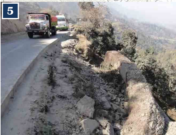
Valley side slope that is deformed and dangerous
