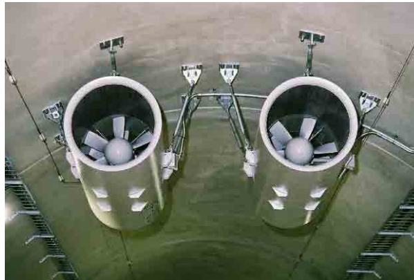
JET FANS INSIDE TUNNEL
