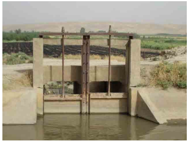
Intake gate on irrigation canal, Kurdish area
