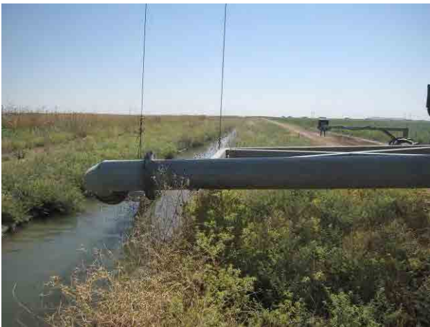
Intake part of the sprinkler system, North Jazira Irrigation Project Area
