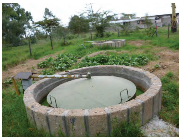
2 nos of digester (100m 3 x 2)
