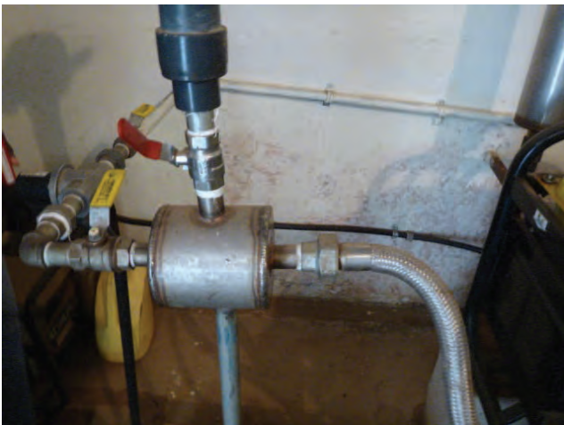
Inlet Gas/Air Valve
