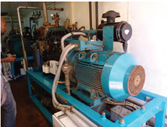
Diesel generator 75 kW x 2
