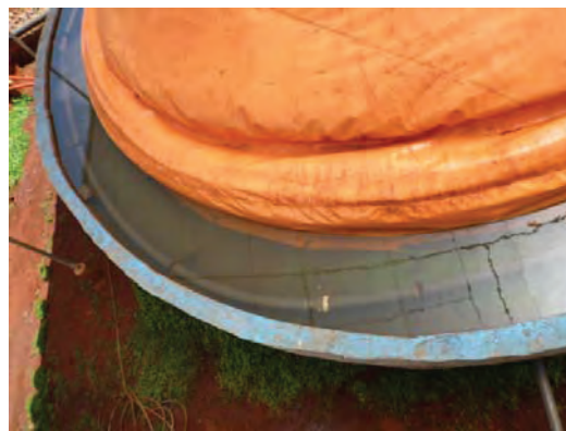
Plastic gas dome and PVC pipe in a pool for gas cooling
