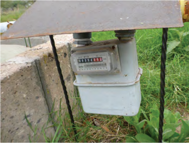
Gas meter at outlet of the digester
