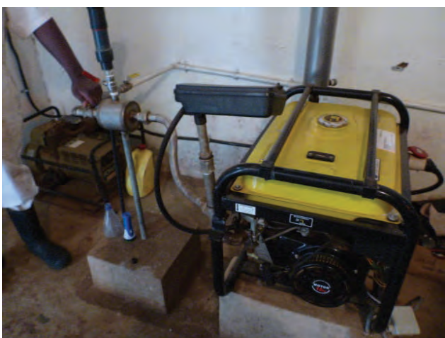
Petro Engine Generator
