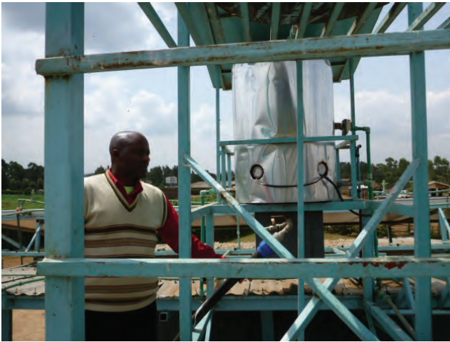
Water Heating for Gas Digester
