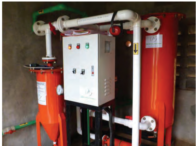
Gas purification unit
