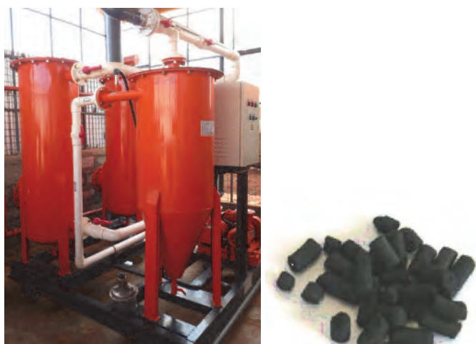
Photos Biogas Filter and Activated Carbon Pellets
