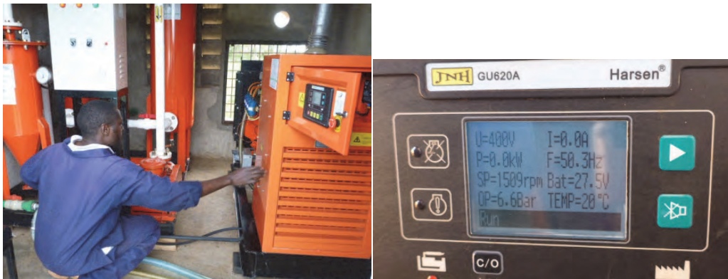
Photos Biogas Generator and Control Panel
