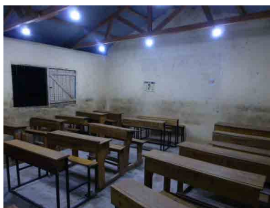
Classroom 1 (with Installed Lights)
