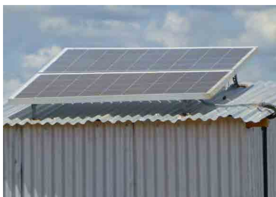
PV Array for Charging House (240 W, DC 12 V) (facing North)
