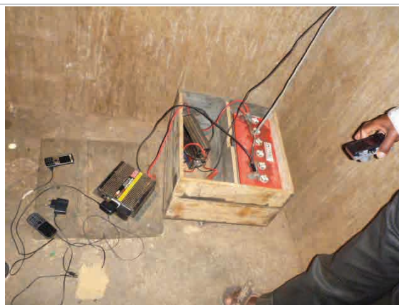
Battery, 600V Inverter and Mobile Charging
