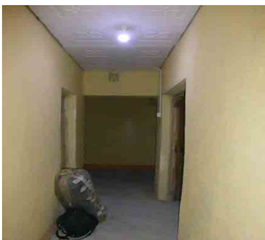
Corridor Light at Latakweny Dispensary
