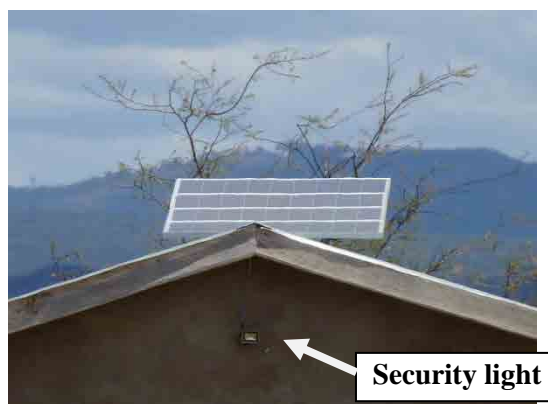
480 W System (DC 24 V) PV Array facing North
