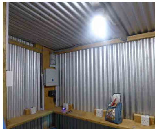
Inside Charging House after Installation
