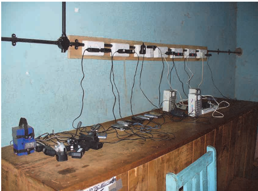
Power outlets on the wall and a shelf are convenient for the operation.
