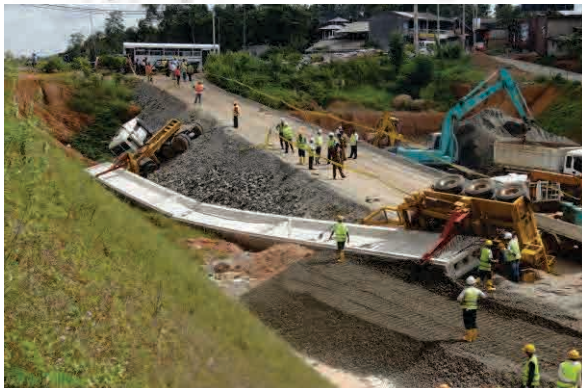
Accident View – looking from the south to the north
