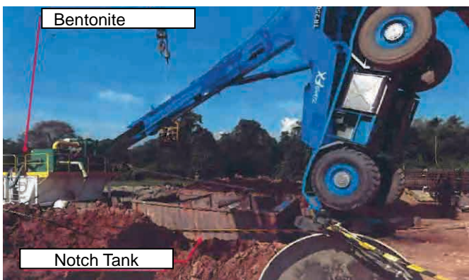
The crane position after topple
