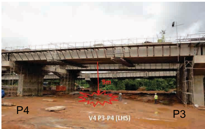
Photo 4.4.3 View of the Accident site
