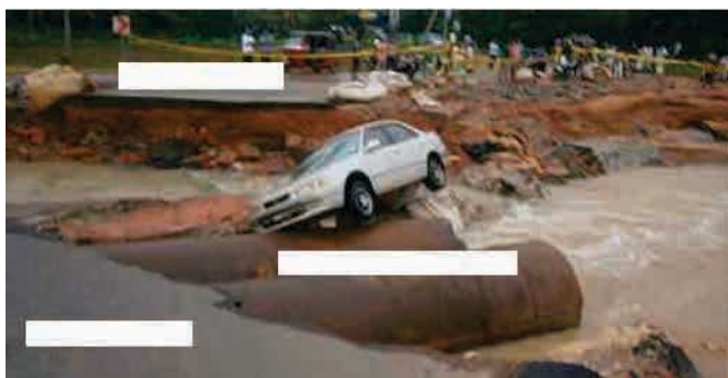
The car which fell on to the pipe culvert. (The situation 4 hours after the incident)
