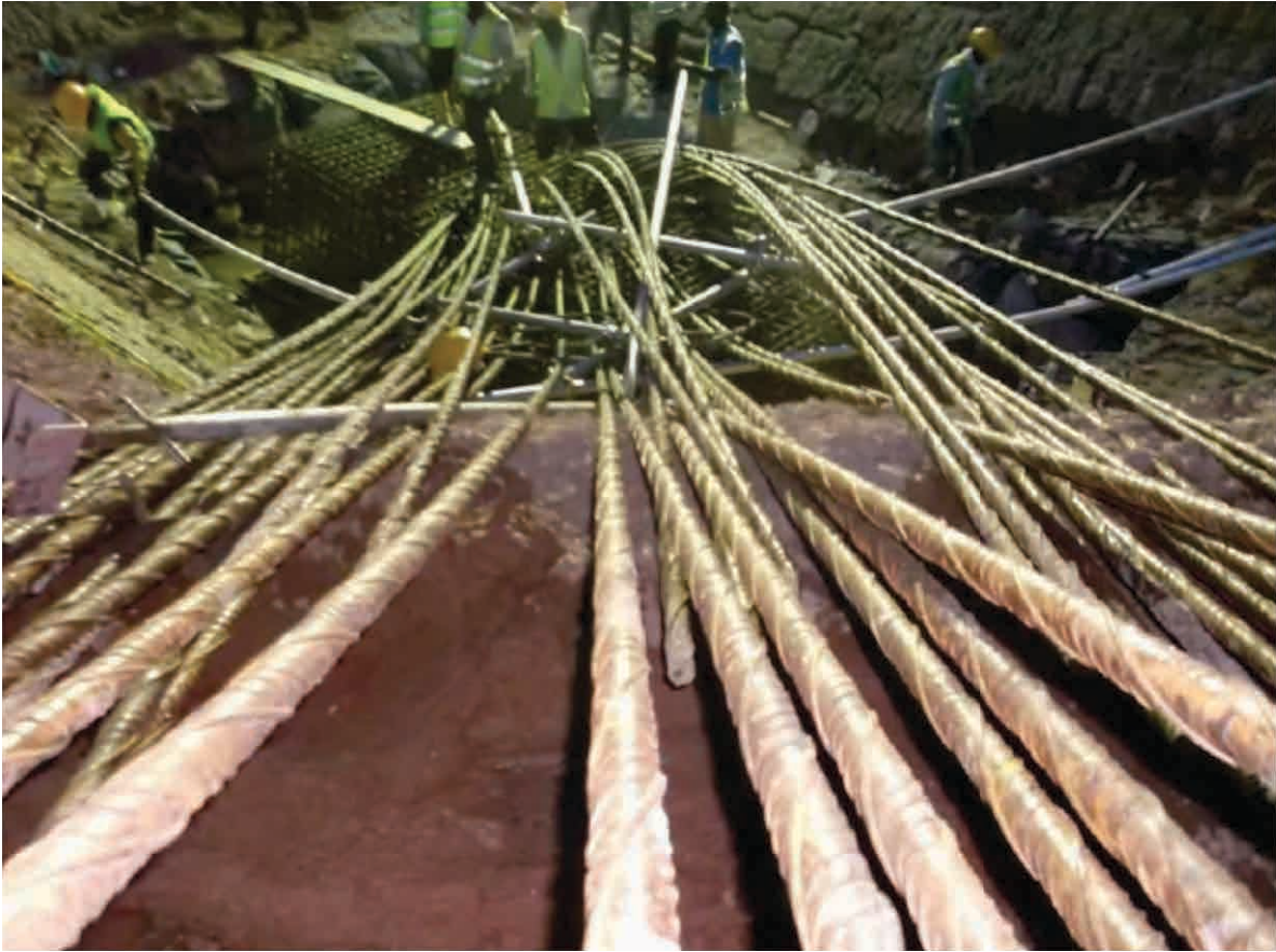
Photo 4.4.7 Tilted Rebar Cage
