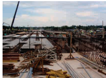
Safety Fence and Net
