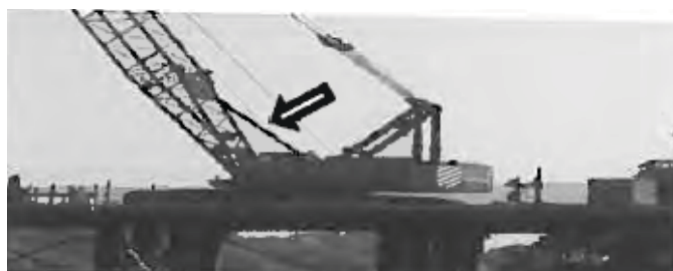
Photo 4.4.1 Crane without stopper
