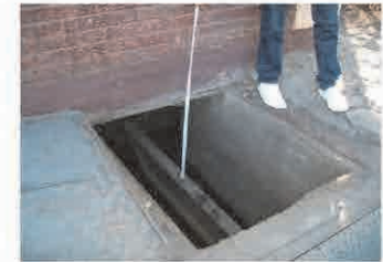
Since drainage pipe is set 30cm below GL (too shallow), drainage pump is used in rainy season (Scale linkage is set 70cm below GL)
