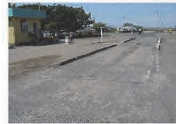
Truck scale and control house
