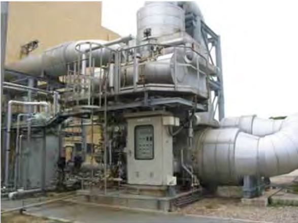
Exhaust gas boiler
