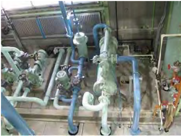
Fresh water intercooler / Primary cooling water pump
