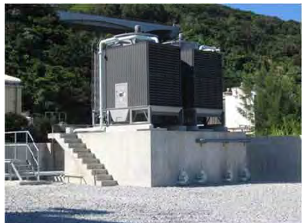
Cooling tower (1000KW Class)
