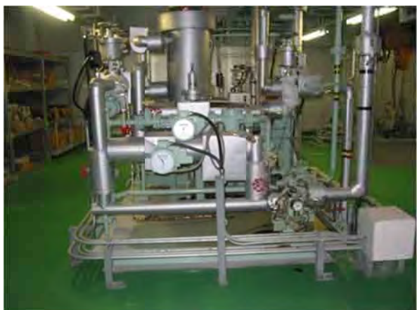
A Class and C class fuel oil meter, mixer and heater
