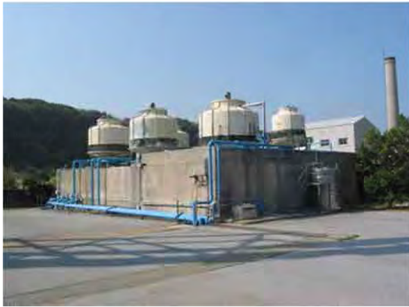
Cooling tower (2500KW Class)
