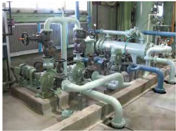
Secondary cooling water pump
