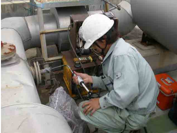
Exhaust gas NOx measurement
