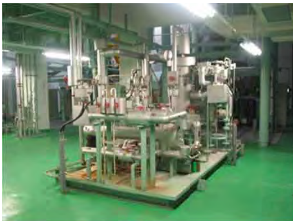
Fuel oil equipment
