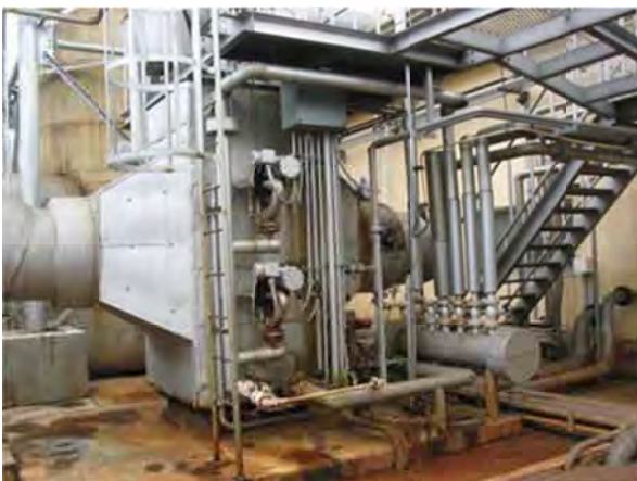
Exhaust gas boiler
