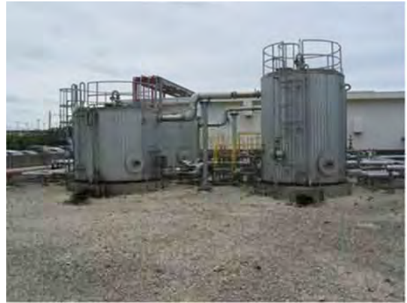
Settling (left) & Clean tank (right)
