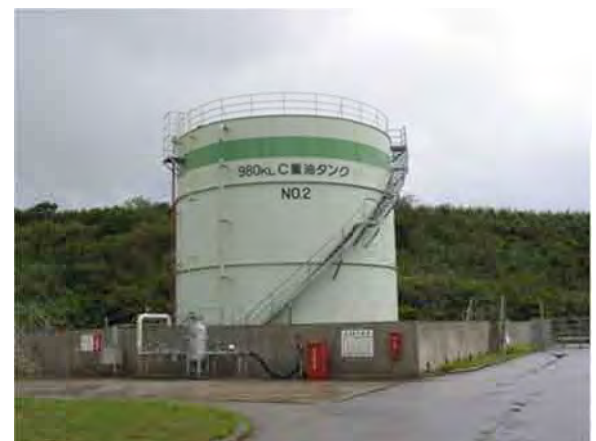
Fuel storage tank (C class heavy oil)
