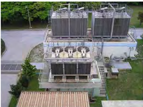
Cooling tower (2000KW Class)
