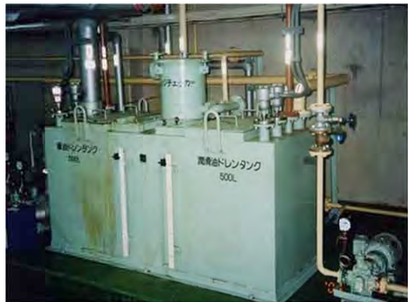
Wastes oil drain tank
