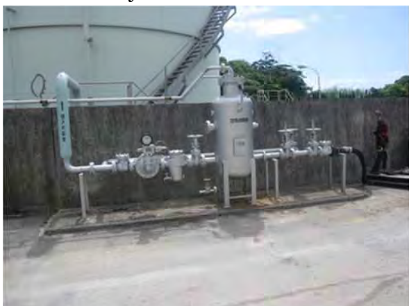
Fuel receiving facilities (air separator, filter, and flow meter)
