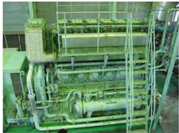
Lubricant oil filter (left side)
