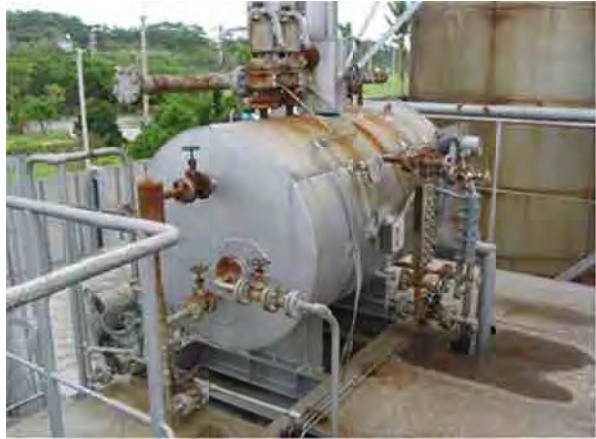
Exhaust gas boiler collector
