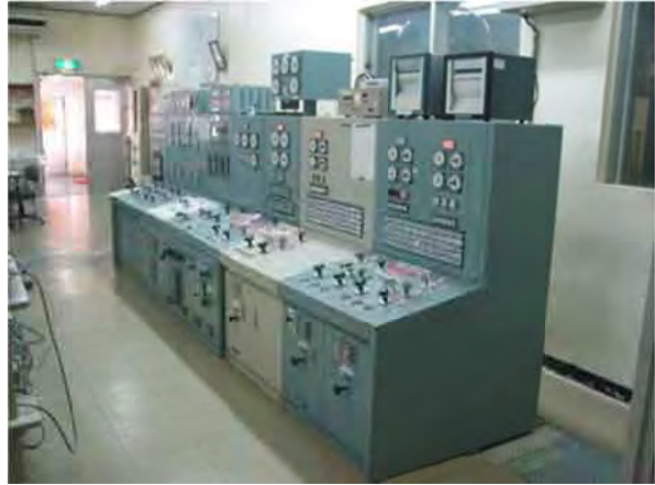
DG Control board
