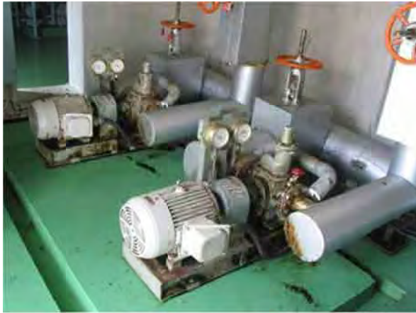
Fuel dispatching pump
