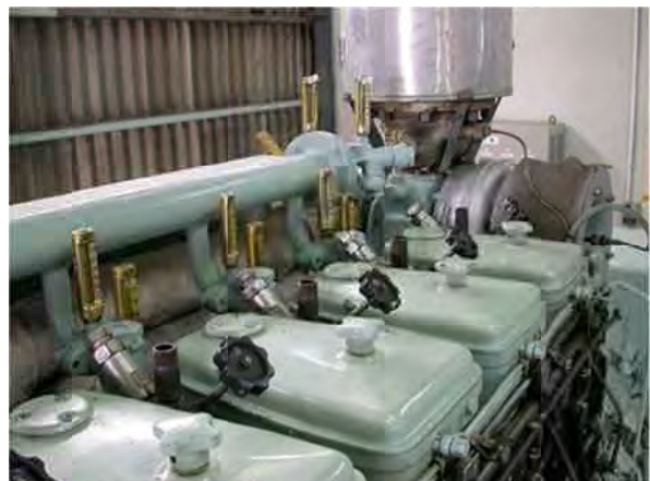
Cylinders head cooling water line
