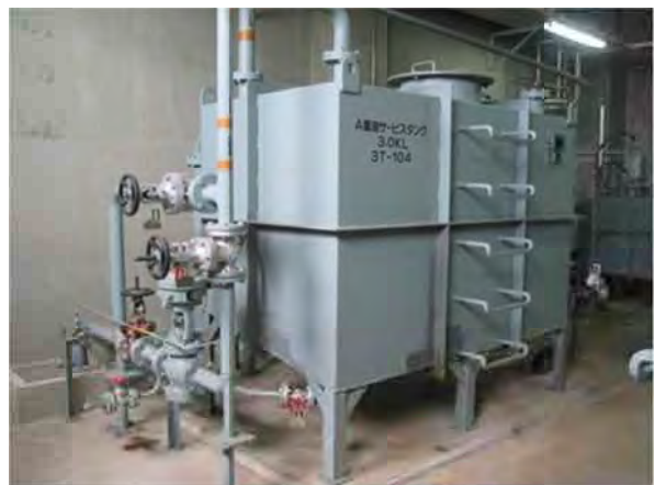
A Class heavy oil daily tank
