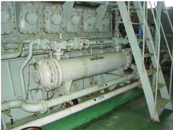
Lubricant oil cooler
