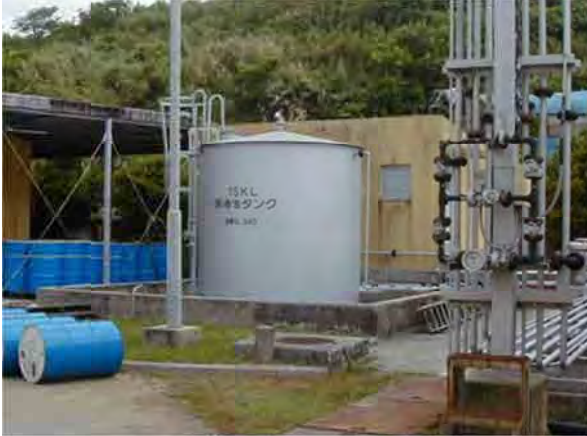
Lubricant oil storage tank
