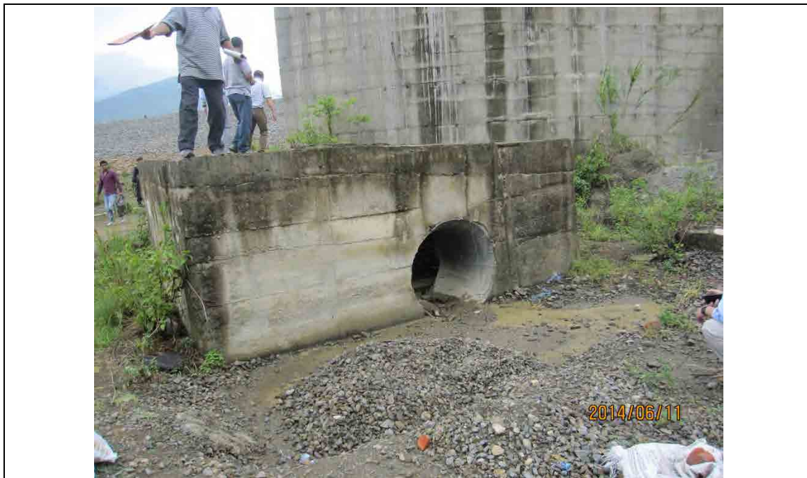
Upper Intake Mouth for Raw Water at Thoubal Dam
