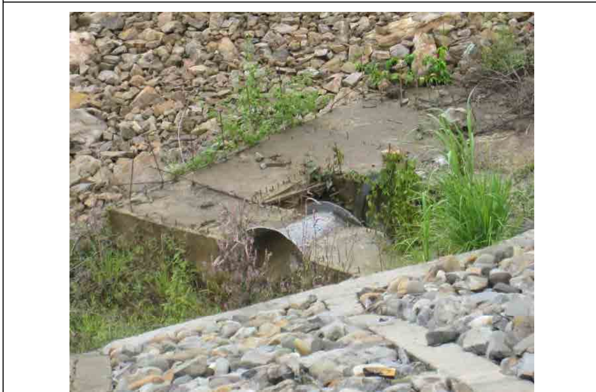
Middle Intake Mouth for Raw Water at Thoubal Dam
