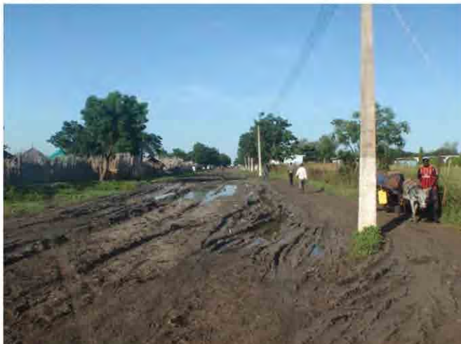
In the rainy season, most of the community roads become impassable.
