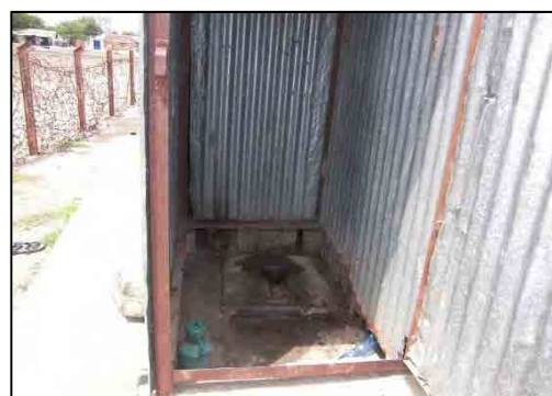
Inside Toilet in Shabia Girl Nation
