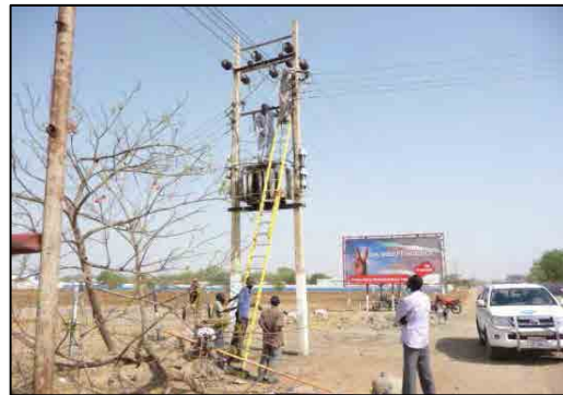
11kV Distribution Line
