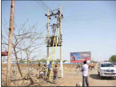
11kV Distribution Line
