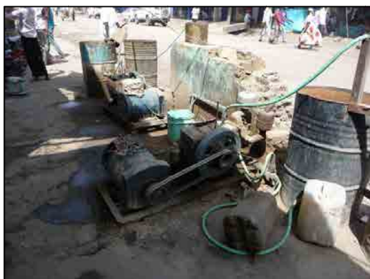
Own Generators in Market
