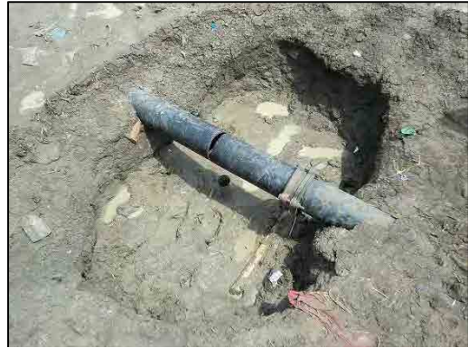
Water pipes are deteriorated and damaged, resulting in high ratio of non-revenue water
