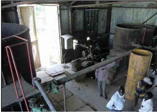
Water Treatment Plant of SSUWC (Filter Tank)
