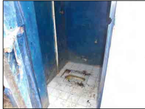
Household (relatively high class) in Hai Television area (Photo shows private toilet)
