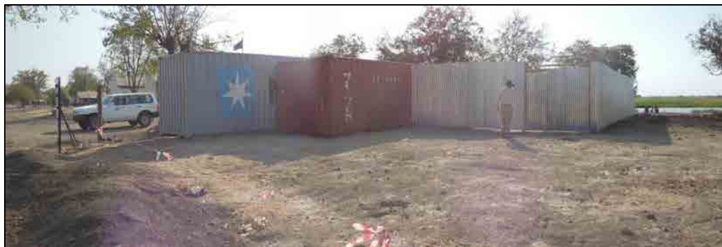
After Leveling of the Ground, Removal of the Facilities and Storage of the Equipemnt and Construction Materials
