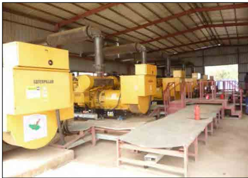
Diesel Generator Engine of Malakal Power Station in Operation
