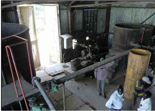
Water Treatment Plant of SSUWC (Filter Tank)
