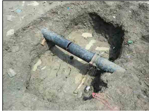
Water pipes are deteriorated and damaged, resulting in high ratio of non-revenue water
