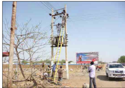
11kV Distribution Line
