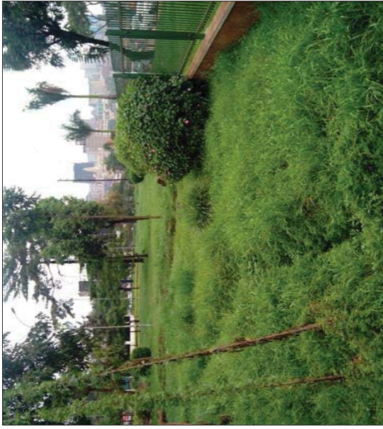
Drainage channel over-grown with weeds at the planned site of the substation extension
