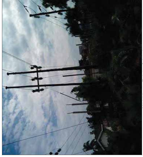
33kV line to Existing Substation
