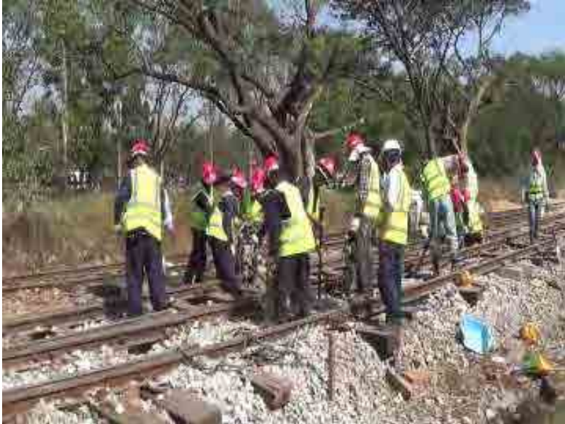
Study for Safety Operation and Management of Railway in the Republic of Ghana 2012 to 2013
