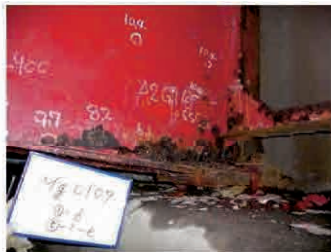
Corrosion of beam end
