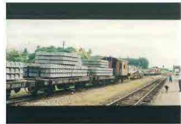
PC sleepers were transported by the trolleys to the site.(Example of Thai railways' rehabilitation works)
