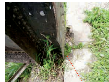
Broken Parapet by Shoe movement
