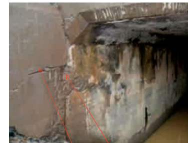
Big crack Flaking
