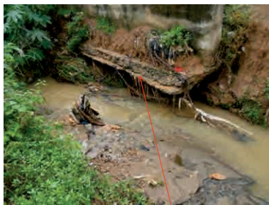
Scouring (Retaining wall)
