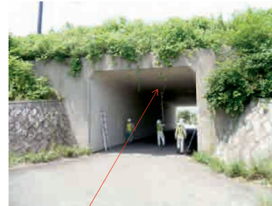
Chalking of crack
