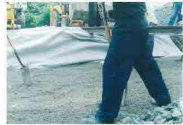
Sand was leveled by the workers. (Example of Thai railways' rehabilitation works )
