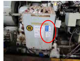
Name tag, Responsible for Daily Maintenance
