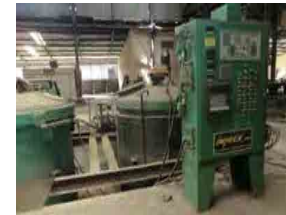
Maintenance facility in an unusable condition
