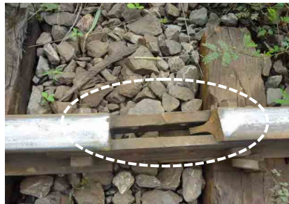
Joint gap is wider than 100mm, and end of right side rail is chipped( Kojokrom ~ Angu section)
