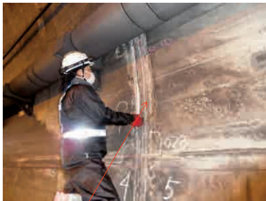
Chalking of crack
