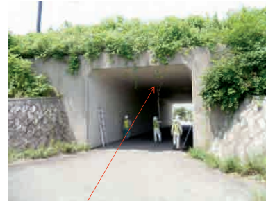
Chalking of crack
