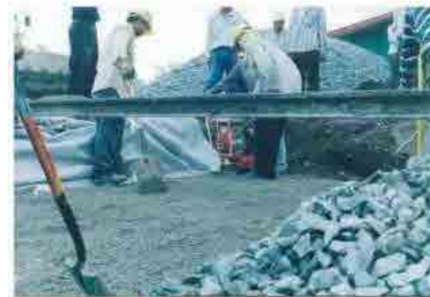
Sand was leveled and tamped by vibration equipment. Water stopping sheet was spread under the sand.(Example of Thai railways' rehabilitation works )
