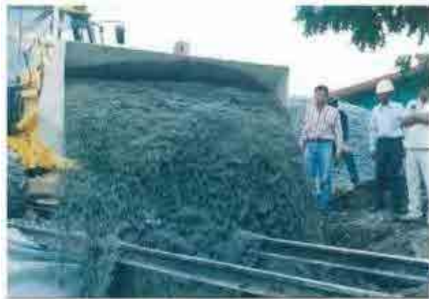
In the rehabilitation work of Thai railways, sand was used as the sub ballast
