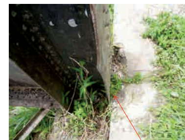
Broken Parapet by Shoe movement
