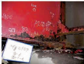
Corrosion of beam end
