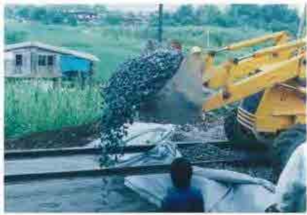
Ballast was installed after finishing sub ballast work.(Example of Thai railways' rehabilitation works )
