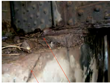
Soil deposits Big crack
