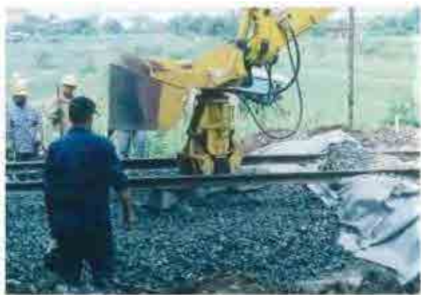
Concrete sleeper (Two block concrete sleeper type, not PC sleeper) was installed by the concrete sleeper renewal machine after finishing ballast work. (Example of Thai railways' rehabilitation works )
