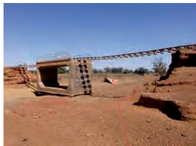
Scouring (Box culvert) In Burkina Faso
