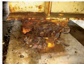
Corrosion of shoe
