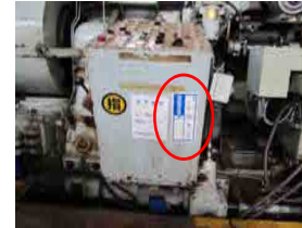
Name tag, Responsible for Daily Maintenance
