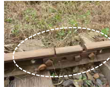
The rail joint structure is not correct (Dunkwa ~ Awaso section)
