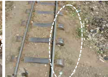
Ballast under the sleeper is too short and width of formation does not measure to standard (Takoradi ~ Kojokrom section)
