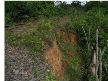
Deep landslide collapse
