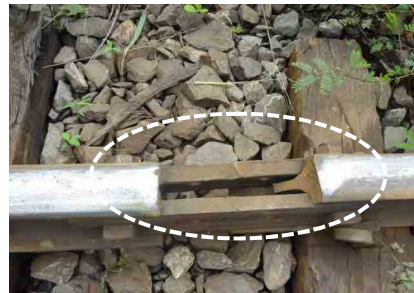
Joint gap is wider than 100mm, and end of right side rail is chipped( Kojokrom ~ Angu section)
