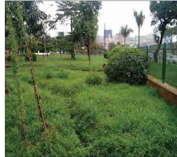
Drainage channel over-grown with weeds at the planned site of the substation extension
