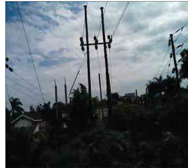
33kV line to Existing Substation
