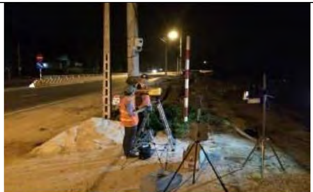
Ph-16 Connecting point with National Route 18 (in QN Province) Noise and vibration measurement (at night)
