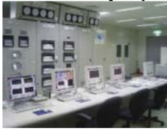
Figure A1.1-3 Central control room
