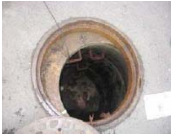
Figure 2.38 Offset of manhole block
