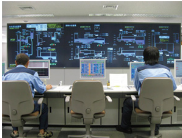
Figure A1.1-4 Main monitoring room in water reclamation centre
