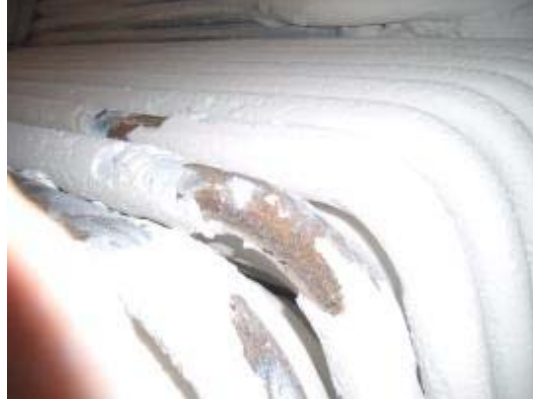
Figure 5.4 Silicon dioxide deposits on boiler tubes
