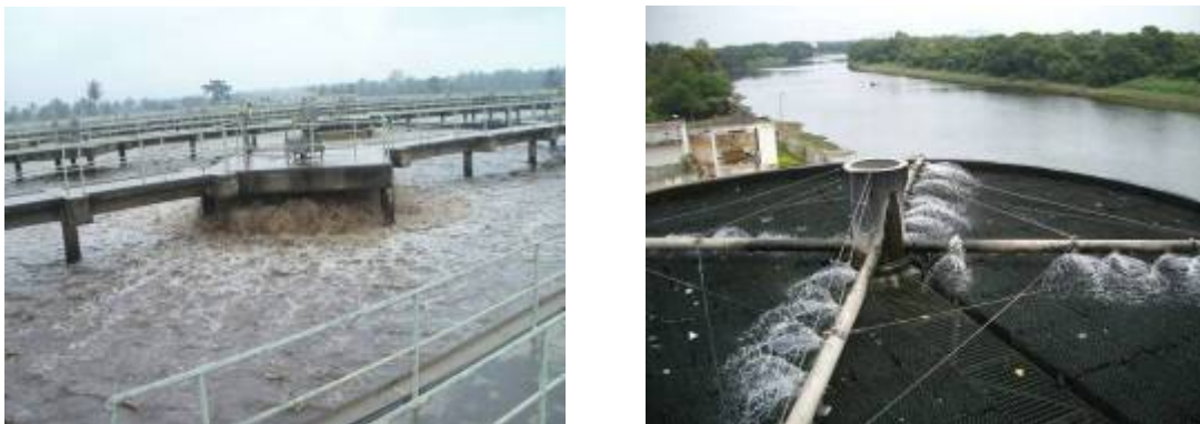
Figure 8.5 Aeration tank (left) and Attached growth system (right)
