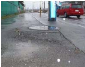
Figure 2.39 Not coinciding with height of road surface
