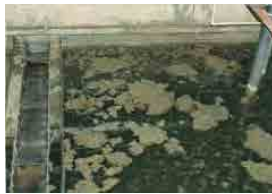
Floating scum in final sedimentation tank in Japan
