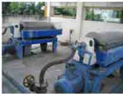
Centrifuge for dewatering
