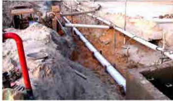
Figure 3.45 Typical arrangements for laying sewers in high subsoil locations using dewatering pump sets, tube wells and Venteak piles with cross brace and nylon rope wrapping around the sewers securing it to the venteak piles and brace
