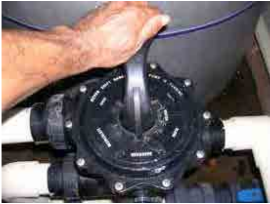
Pic10 Select the backwashing mode in the sand filter controller.
