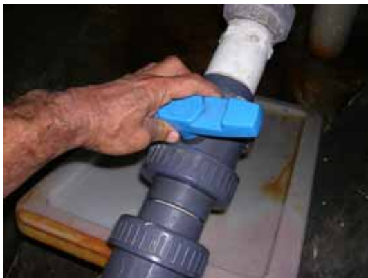
Pic5 Close the stop valve for the seawater intake pump.
