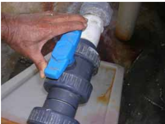
Pic11 Fully open the stop valve for the pump.
