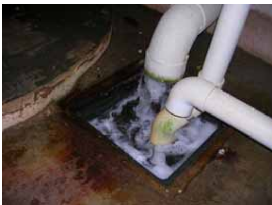
Pic3 Discharge of overflowed water. Now the tanks at the top of the pump house become full.
