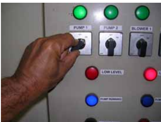
Pic12 Turn on the switch for the pump.
