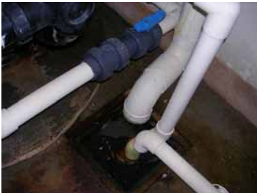
Pic2 4" drain pipe from the elevated water storage tanks appears in the center of this picture taken at the water discharge pit.
