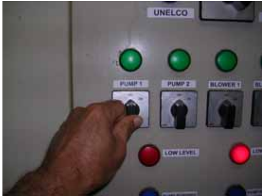
Pic4 This power switch is located on the control panel.
