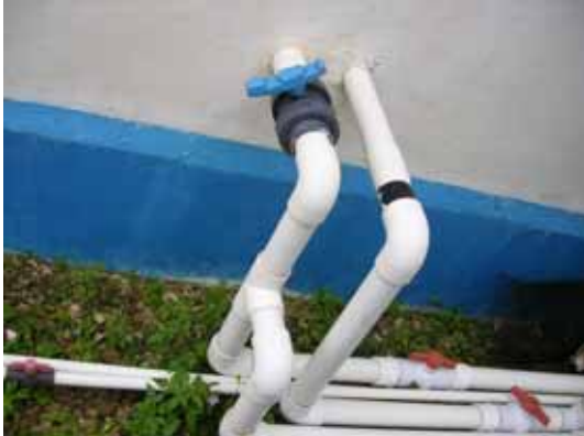
Pic1 The main valve (w/ blue handle) is located outside the pump house.
