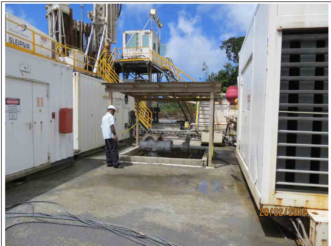
Figure 9. WW-3 Geothermal Well.
