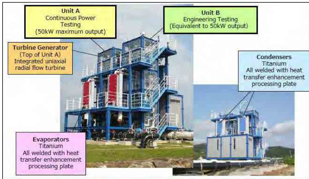
Figure 9 The Installed and Running OTEC Demonstration Facility at the Okinawa Deep Seawater Research Institute (Kume Island)
