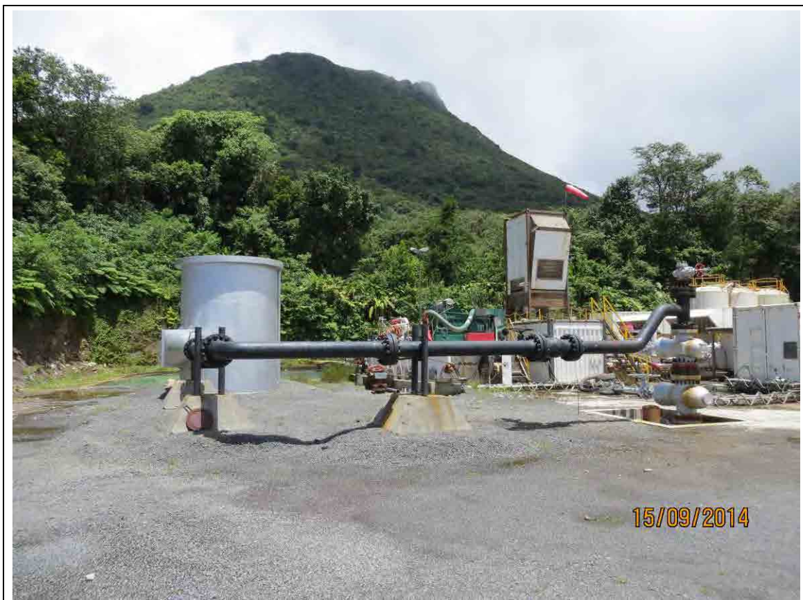
Figure 7. WW-PI Geothermal Well
