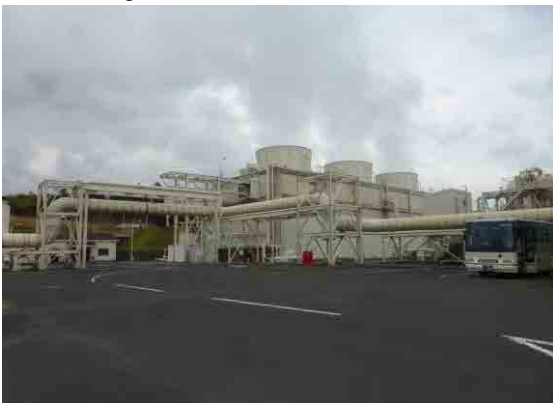
31 October,2014 Exterior of Ogiri Geothermal Power Station
