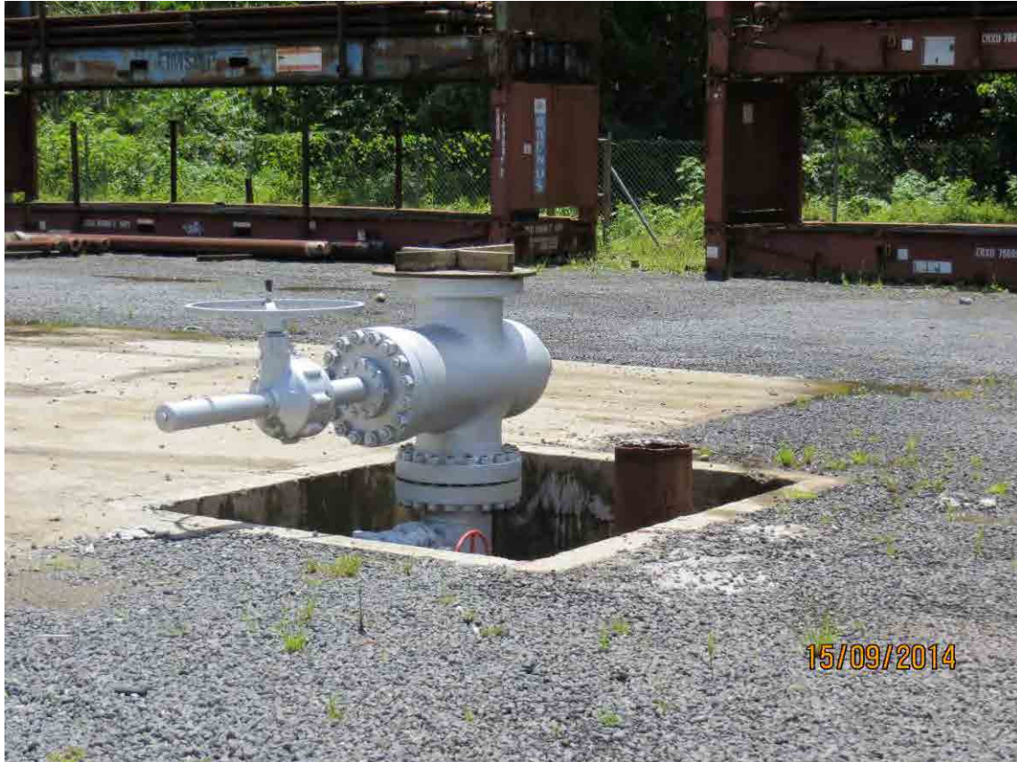
Figure 3. WW-R1 Geothermal Well
