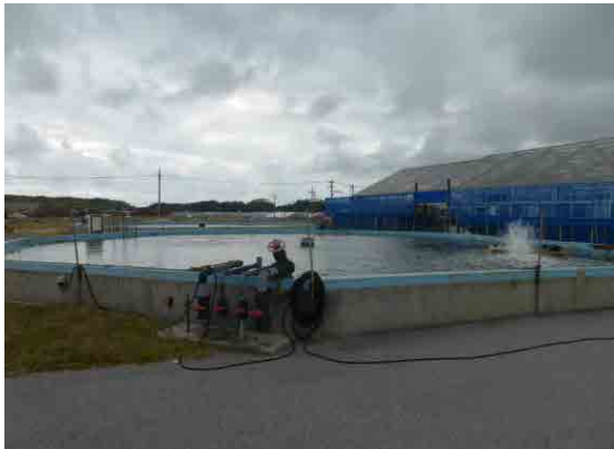
2 November, 2014 Water Storage Facility at Okinawa Deep Seawater Research Center
