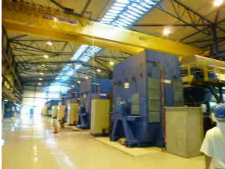
Figure 3 Diesel power plant (St. Lucia)
