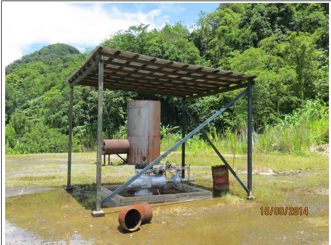
Figure 5. WW-1 Geothermal Well
