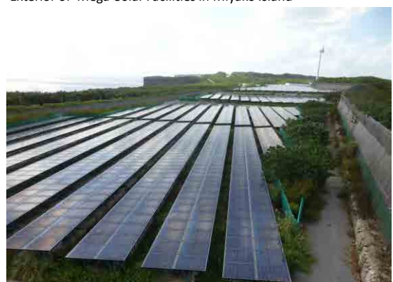
4 November, 2014 Exterior of Mega-Solar Facilities in Miyako Island
