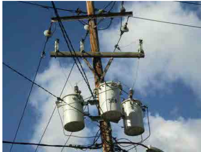
Figure 9 Pole Transformer (Dominica: ABB Production (USA))
