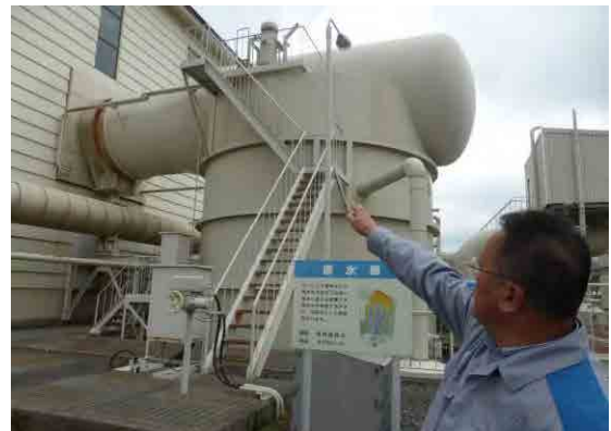
31 October,2014 Facility Tour at Ogiri Geothermal Power Station
