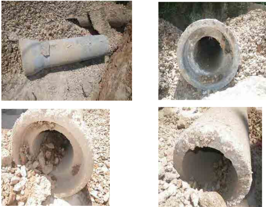
Figure 5.3 Concrete Pipes used in Jordan
