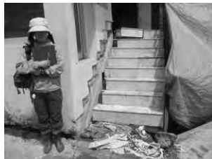
Sinking of steps caused by landslide
