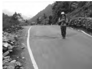
Uneven road caused by landslide
