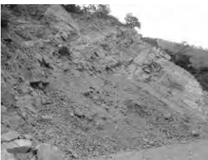
Surface failure and rock fall
