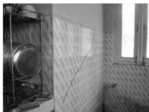
Clack of wall caused by landslide
