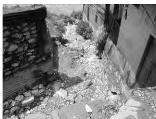
Inadequate channel works
