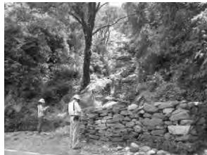
Exit of hillside collapse
