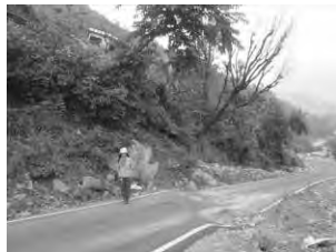
Inclination of house and uneven road
