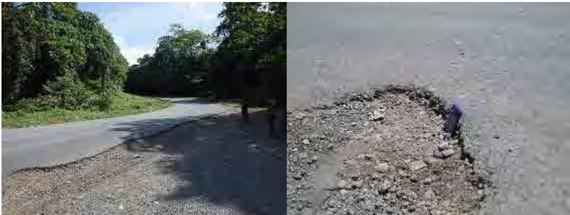
Photograph 2.2.2 Damage to Paving Edges
