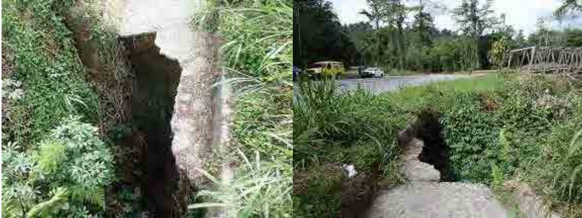
Photograph 2.2.1 Roadside Erosion and Collapse caused by Channel Damage
