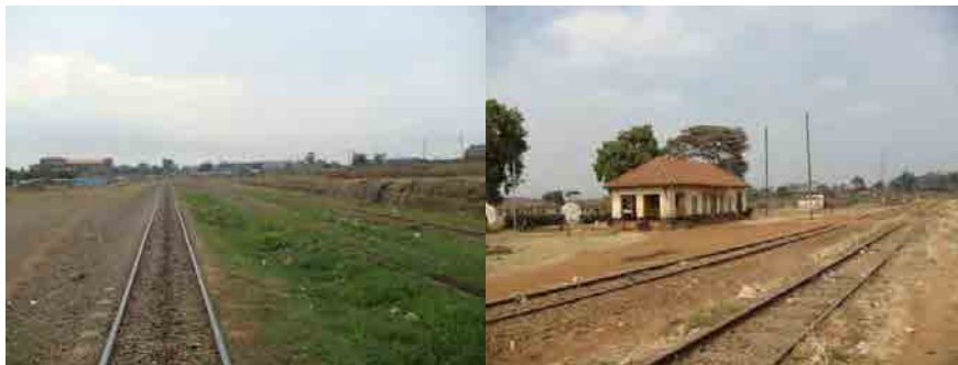
Figure 4.2.6 Existing Track Condition (left), Existing Ruiru Station (right)
