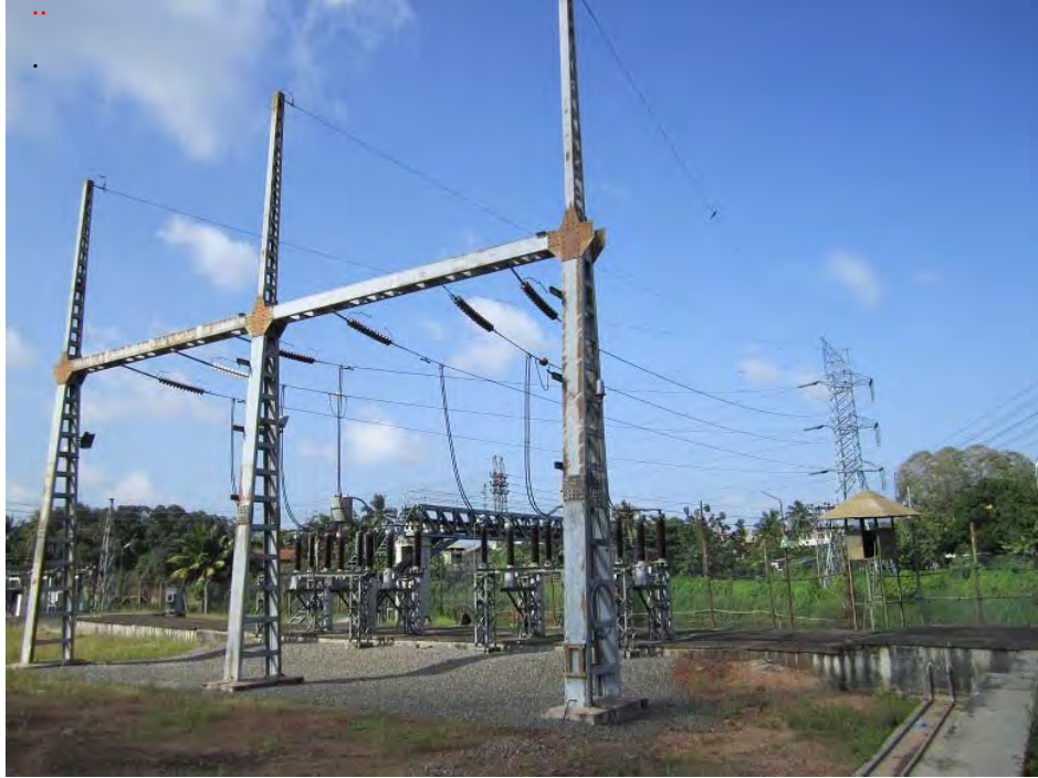
Existing 132kV Kolonnawa– Pannipitiya line and gantry
