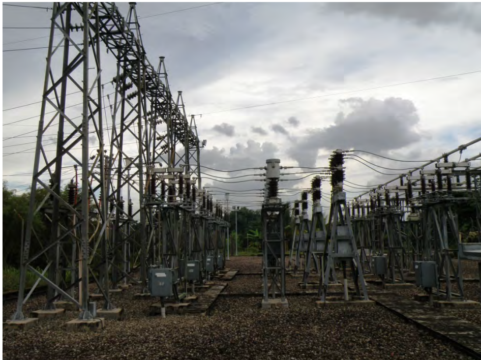
Existing 33kV switchgear (DS, DE/ES) to be replaced
