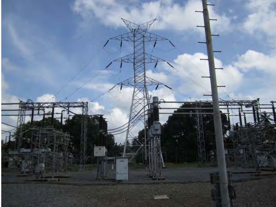
Existing 132kV Ratmalana dead-end tower (It is plan to be removed) and 132kV switchgear to be replaced (CB, DS, CT)
