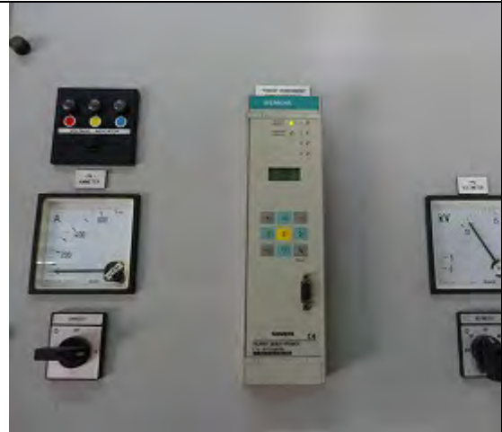
RMU Switch Panel (Circuit Earth fault Relay: Siemens)
