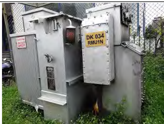
Existing UG transformer.
