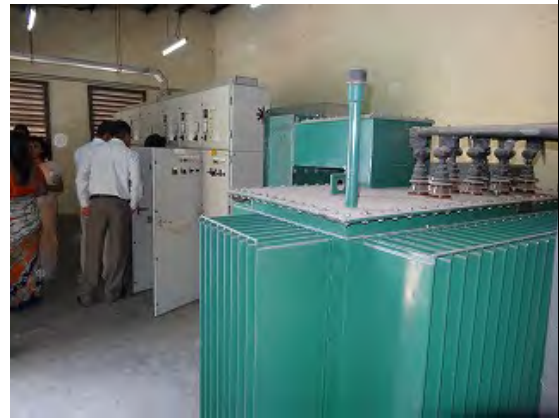
UG Transformer (800kVA) & MV SW Panel
