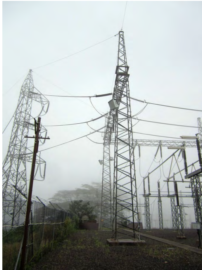
Existing 220kV Switchyard
