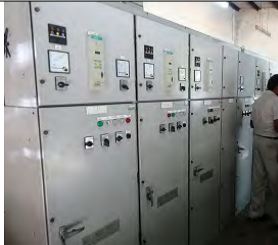
RMU Switch Panel (Vacuum Switch: RANHILL POWER BERHAD )
