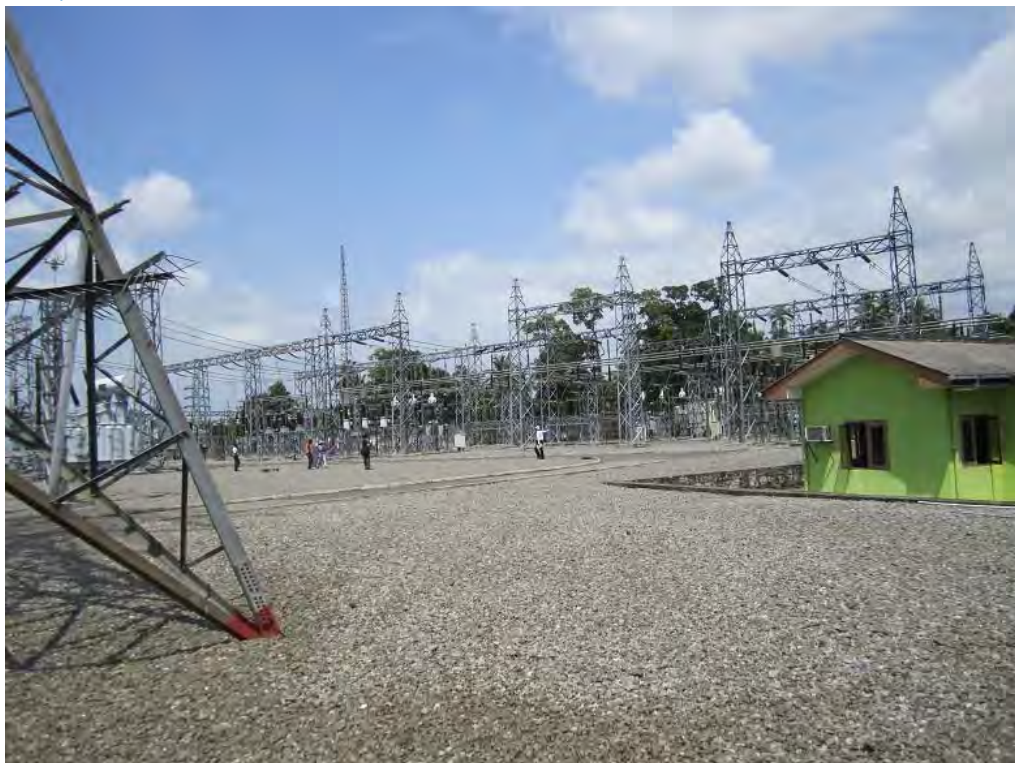
Existing 132kV spare TL bays for Thulhiriya line (Right-end and 3 rd from right, front area of these bays will be used for 220kV new bay)
