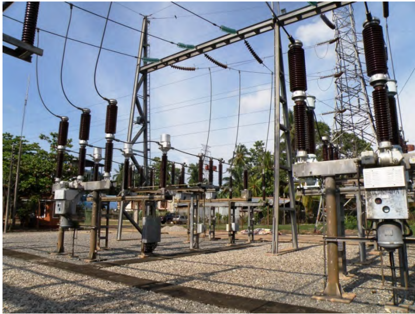
Existing 132kV switchgear (CB, CT and VT) to be replaced
