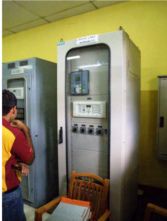
Existing 220kV TL Protection facility to be replaced
