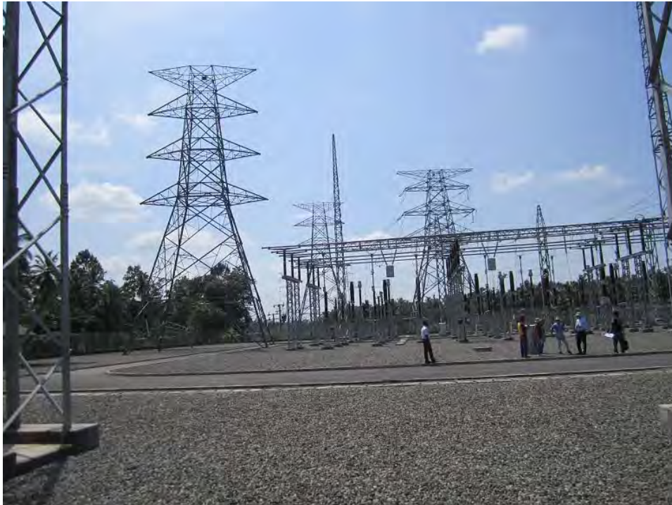
West direction view from 132kV bay (The old 132kV towers needs to be removed and New two 220kV bays will be extended)
