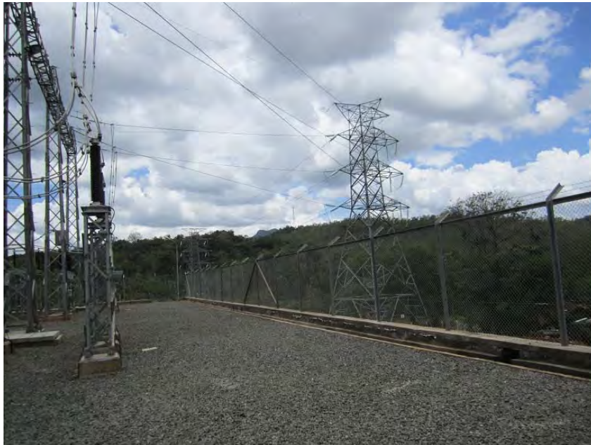
Existing 132kV Naula / Habarana in-out dead-end and second dead-end tower will be used for the new line.
