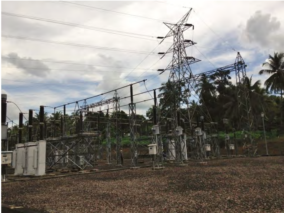
Existing 132kV T/L switch backed and connected to north faced gantry. (New T/L is planned in the same connection style)
