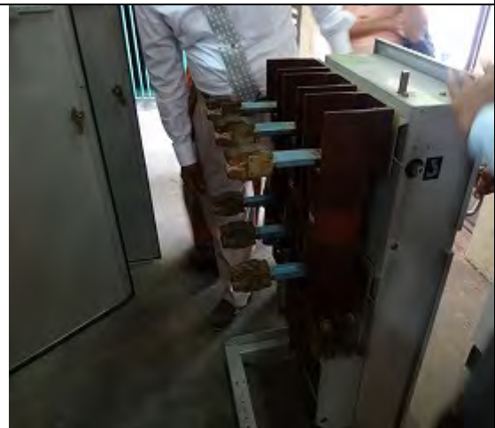
RMU Vacuum switch (RANHILL POWER BERHAD )
