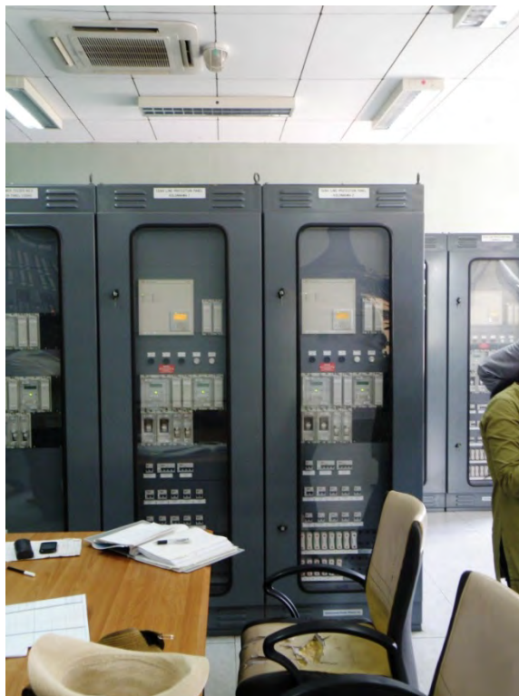
132kV TL Protection facility to be modified
