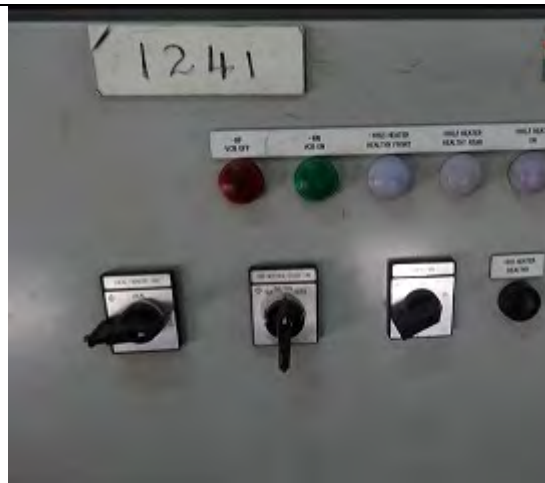
RMU Switch Panel (Controller: RANHILL POWER BERHAD )
