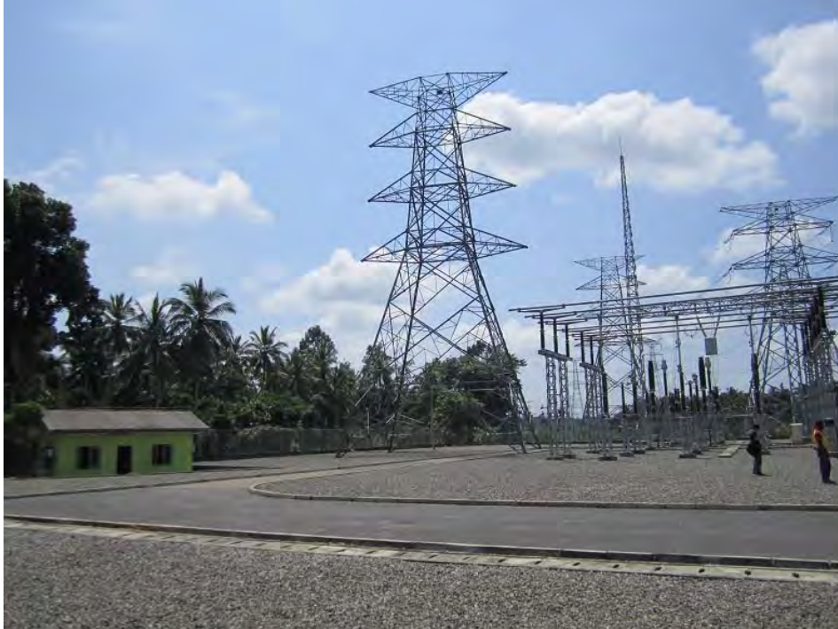
Area for new 220kV bay extension (Old 132kV tower are center and back)
