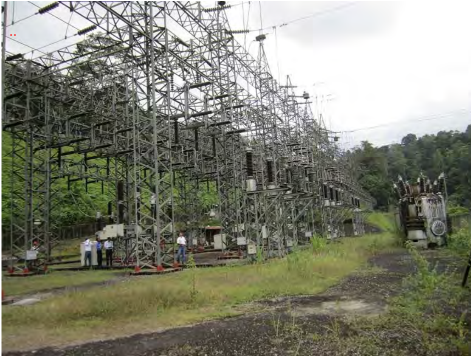
Existing 132kV bay (1 st and 2 nd bay from near side is for new line)
