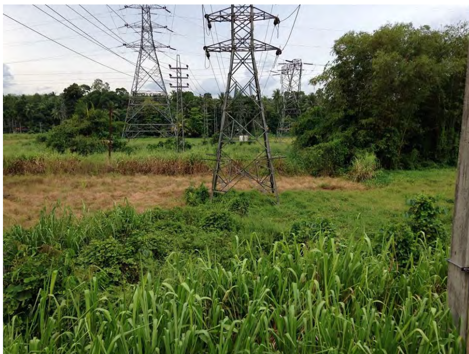
Some 33kV and two 132kV existing T/L are located on south area of GS (New T/L will come from this direction)
