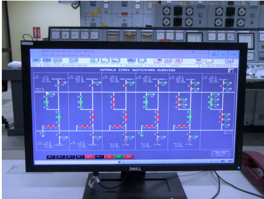
Existing SAS system for 220kV Switchyard
