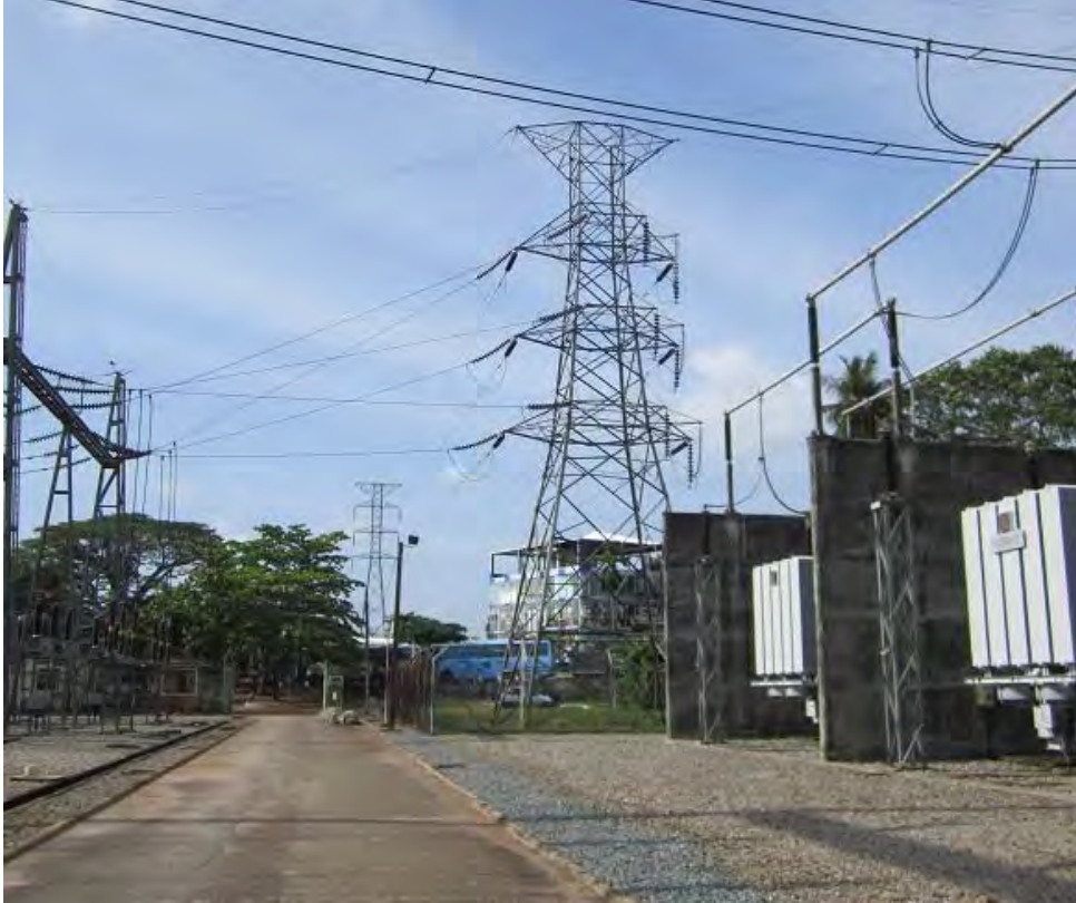
Existing 132kV Kolonnawa– Pannipitiya line (Dead end tower)
