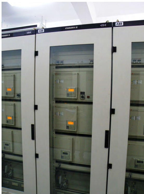
132kV TL Protection facility to be modified
