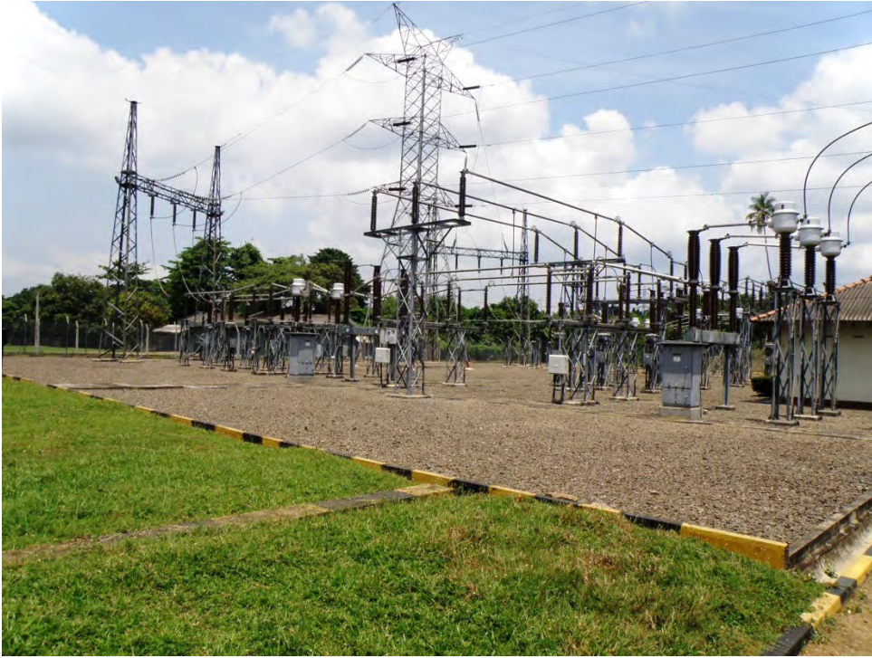
132kV Switchgear equipment to be replaced
