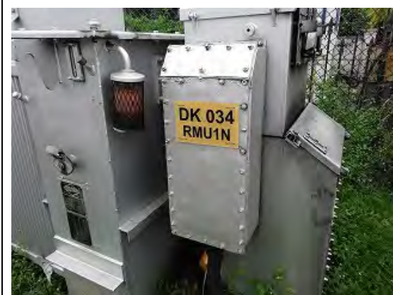
Primary (MV 11 kV) RMU side.
