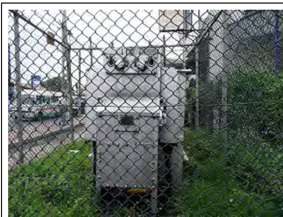
Existing pad-mount transformer.
