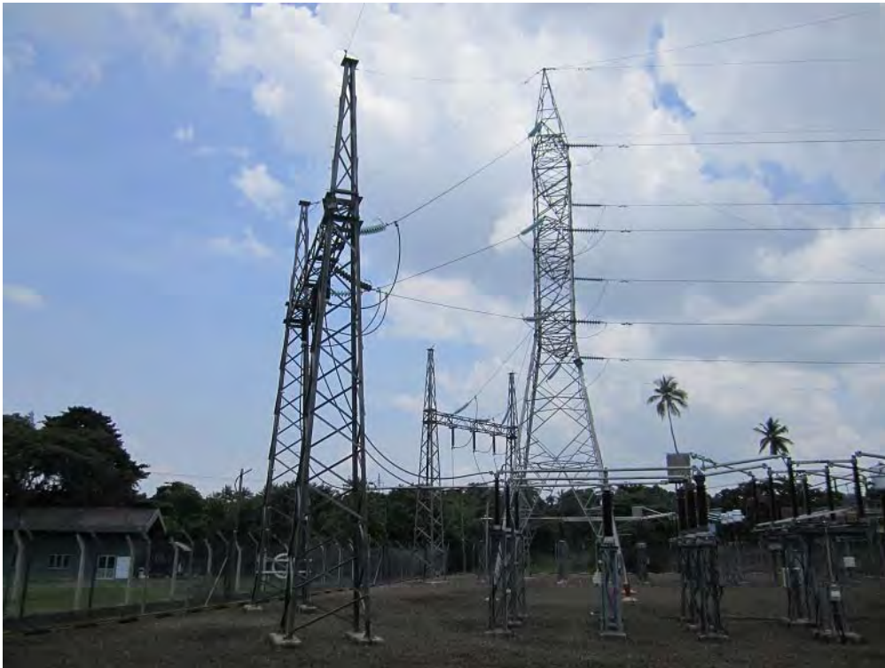
Existing 132kV Polpitiya / Aturugiriya in-out line and gantry
