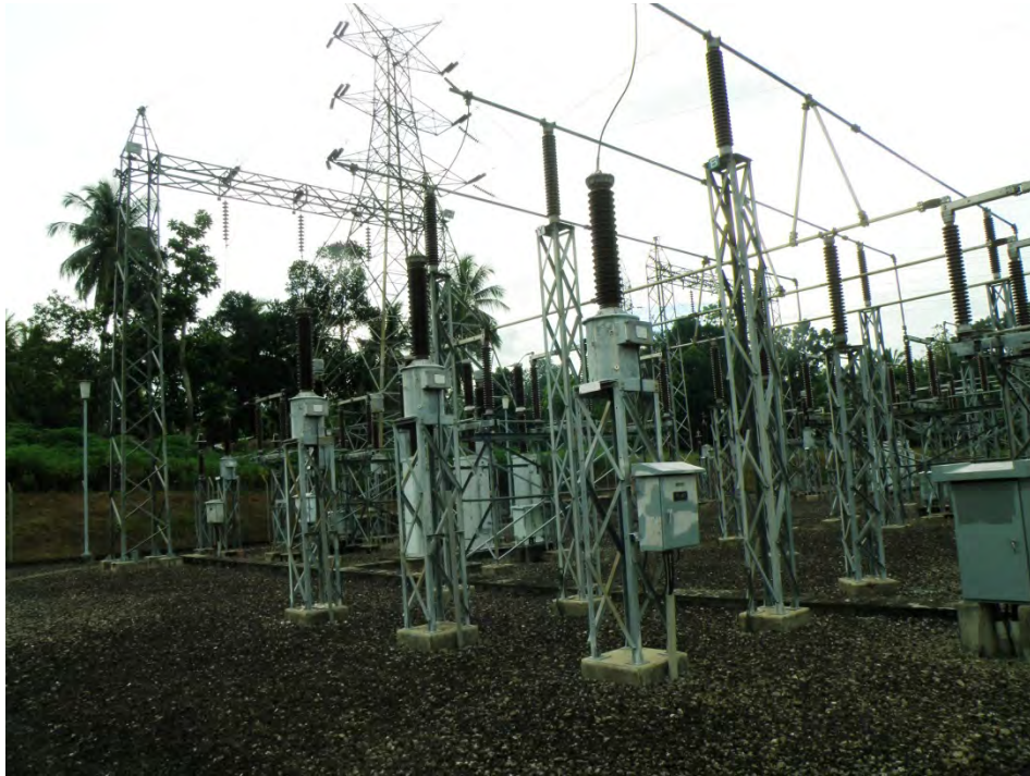
Existing 132kV switchgear to be replaced
