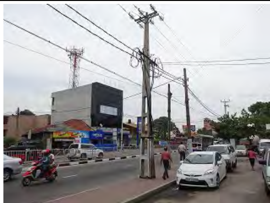
LV power feeding point (LV UG cable from pad-mount Tr along the pole).
