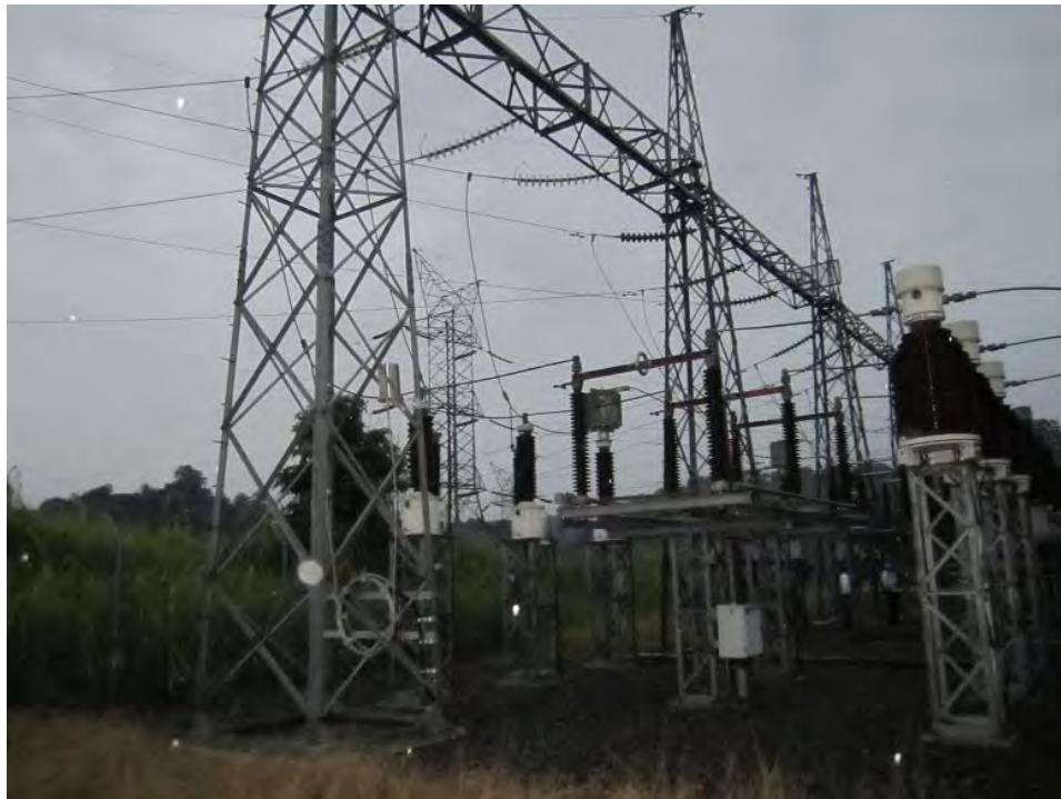
Existing 132kV bay will be used for new T/L
