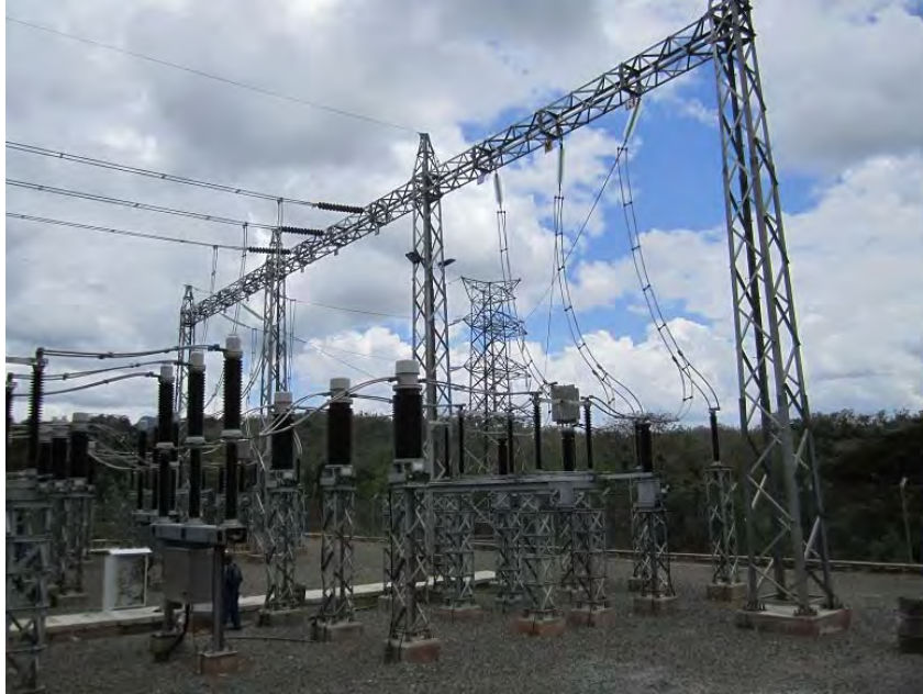
Existing 132kV Naula / Habarana in-out line gantry
