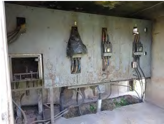
LV switch panel of existing facility
