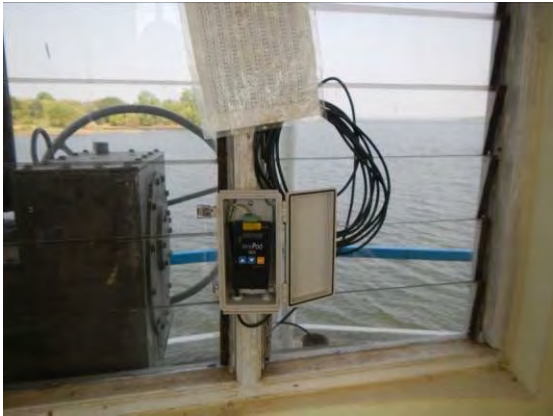
Figure 6-3-9 Water Level Recorder
