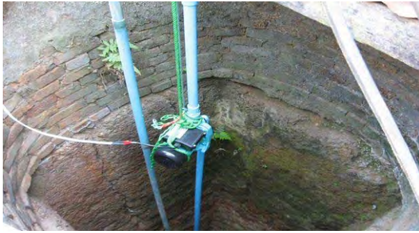
Figure 3-2-13-3 Pump used at Shallow Well
